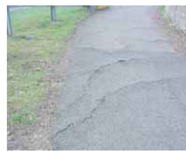
2b Cycle track requires relaying due to damage from tree roots.
