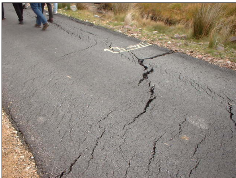
Figure 1.2.1: Example of Deterioration on Low Trafficked Road
