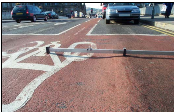
Figure 9.1.1: Example of Rutting
