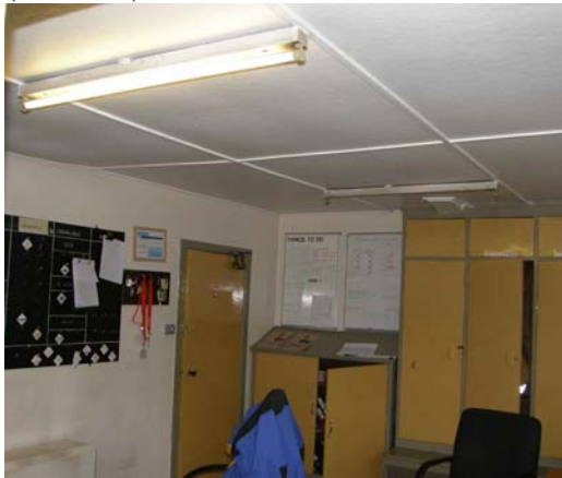
01 - Watch Room lighting
