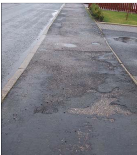
Figure 1.2.1: Example of Surface Deterioration on a Footway
