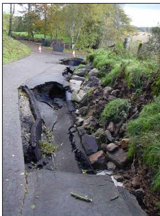
Figure 4.5.1: Flood Damage to Road
