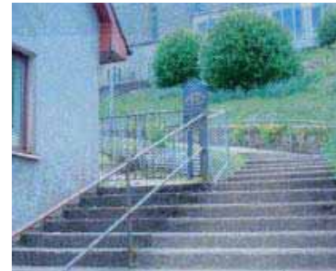
6c The steps provide a good short cut to the town centre. However there is evidence of drinking and urination.
