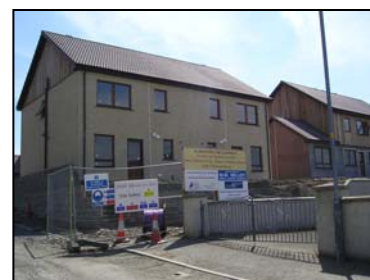
Construction on the Pentland Housing Association development at Harrow Hill, Wick completed in 2006
