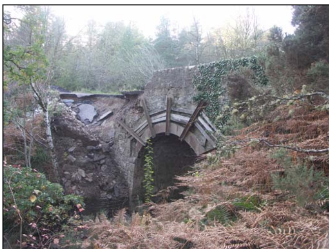
Figure 8.1: Quebec Bridge Flood Damage
