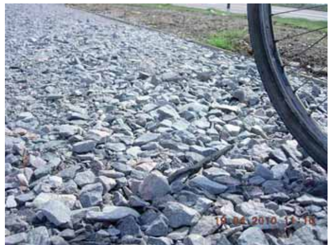
Figure 3-20: Poor quality surfacing on new B817 cycle track
