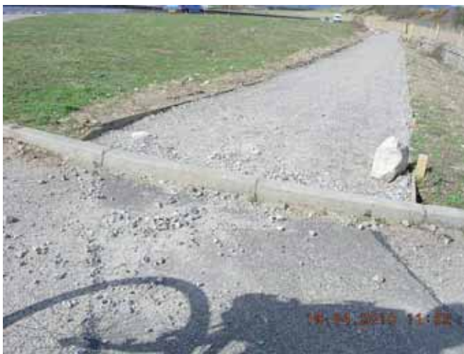
Figure 3-19: No dropped kerbs on new cycle track on B817
