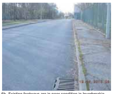
6h Existing footways are in poor condition in Inverbreakie Industrial Estate.
