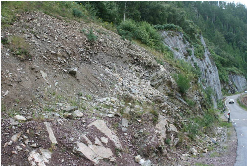
Photograph 10: Possible location of northern portal, further assessment would be required to confirm the angle of entry and the amount of cover rock (currently covered by mesh) that could be retained.
