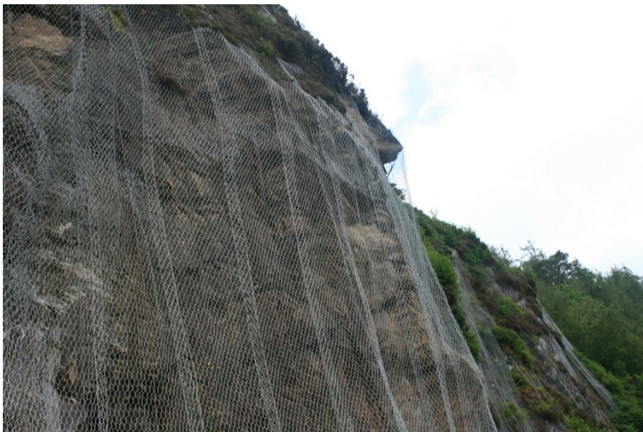
Photograph 7: Example of the netting works undertaken to date along much of the exposed faces adjacent to the A890.
