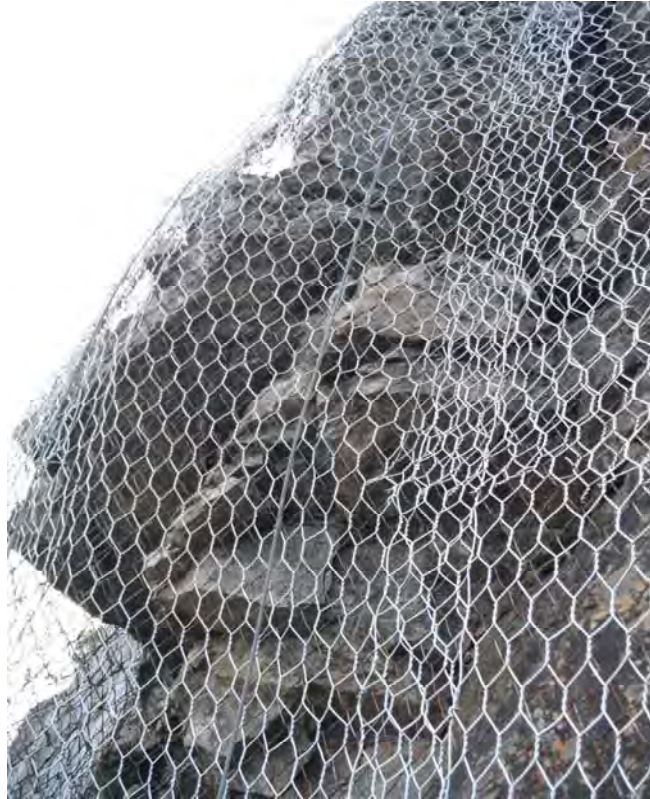
Photo 13: AA22B - 12m 3 'nose' resting on ravelling blocks centred on a poor join in the netting (wire twist joins at 0.5 - 0.7m centres)
