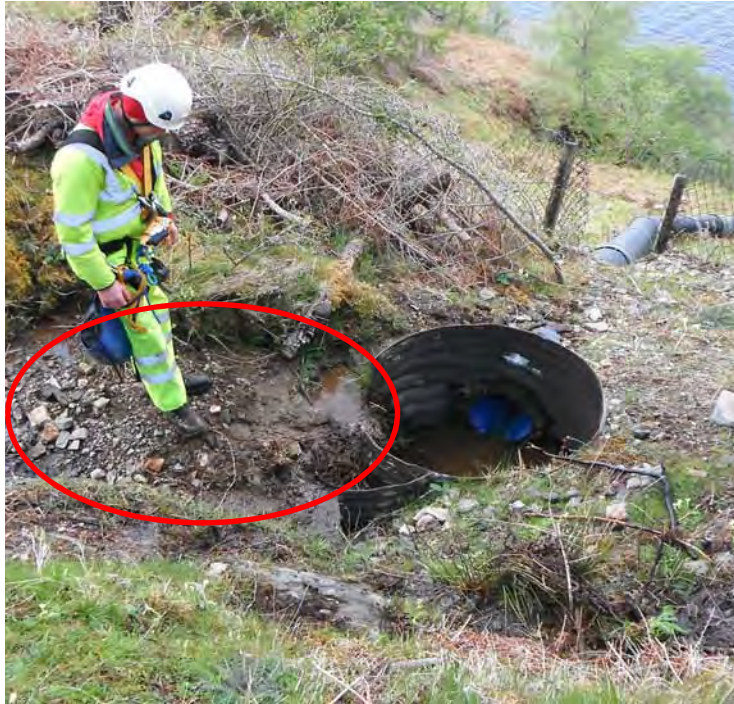
Photo 3: Gully between AA5 and AA6 - End of ditch at catch pit requiring removal of sediment build up to prevent overflowing of water onto slope surface.
