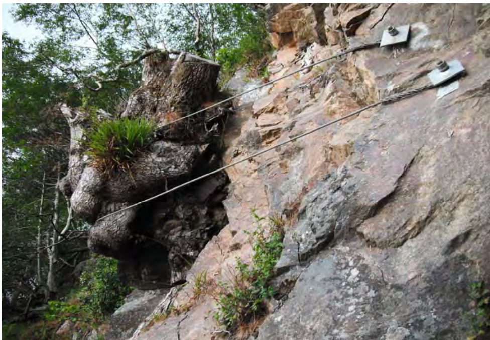
Photo 10: AA19 Upper - 2m 3 dead tree stump and rock blocks with cable straps.
