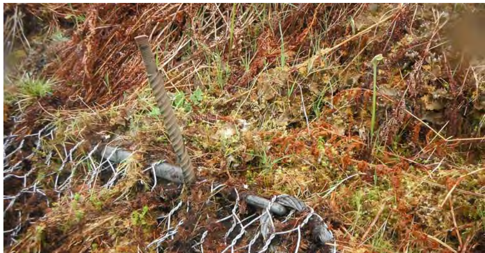
Photo 12: AA17 - Top anchors driven into ground, no evidence of grout.
