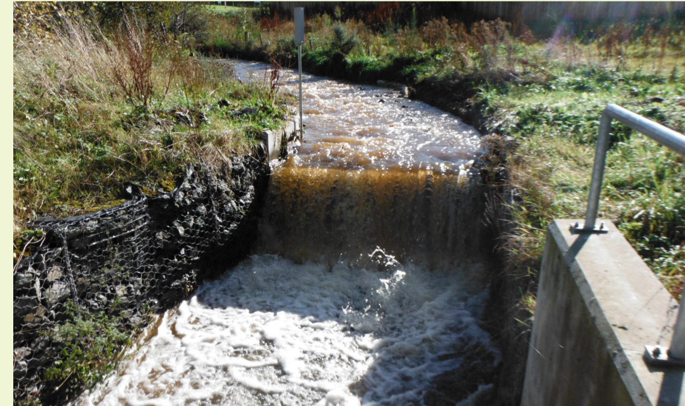
Blocked debris screen
