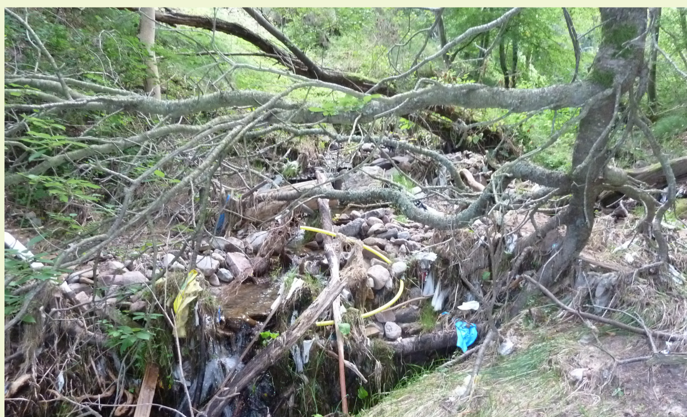
Smithton Burn: debris blockage, upstream of railway culvert
