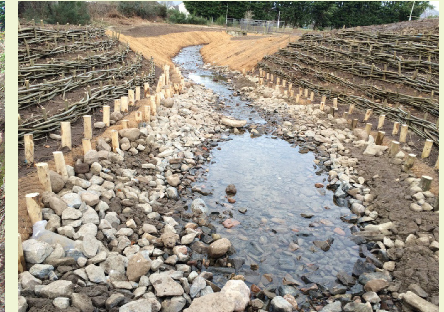
After: Channel re-sectioned to reduce flow velocities and protect the banks using natural 'living' products to stabilise the banks.
