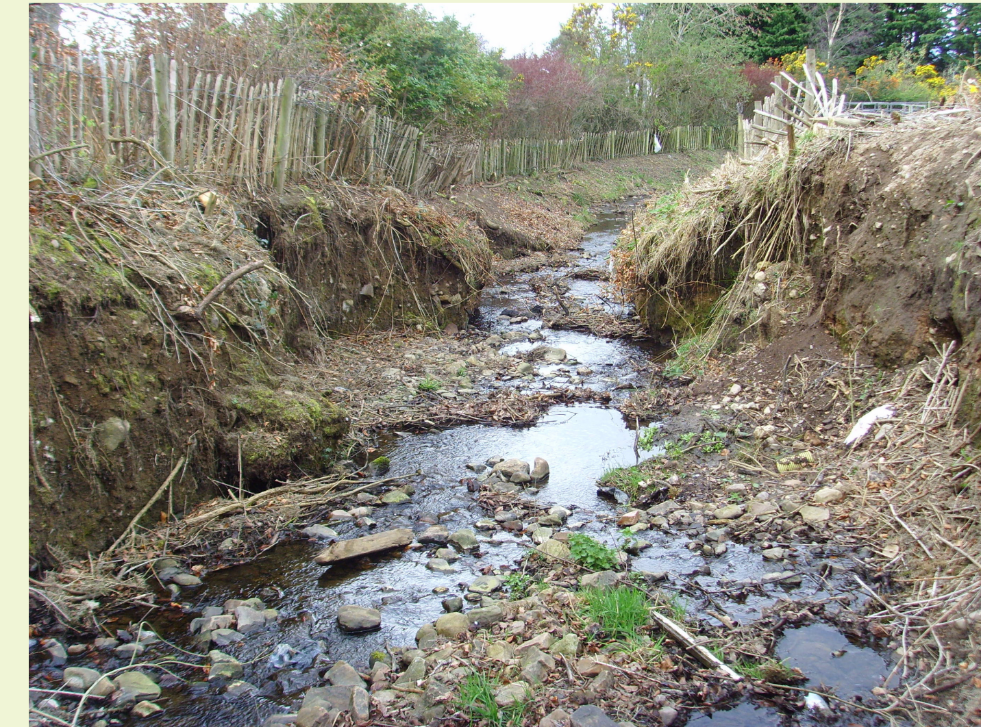
Before: Smithton Burn, with uncontrolled bank erosion increasing the risk of downstream blockage.
