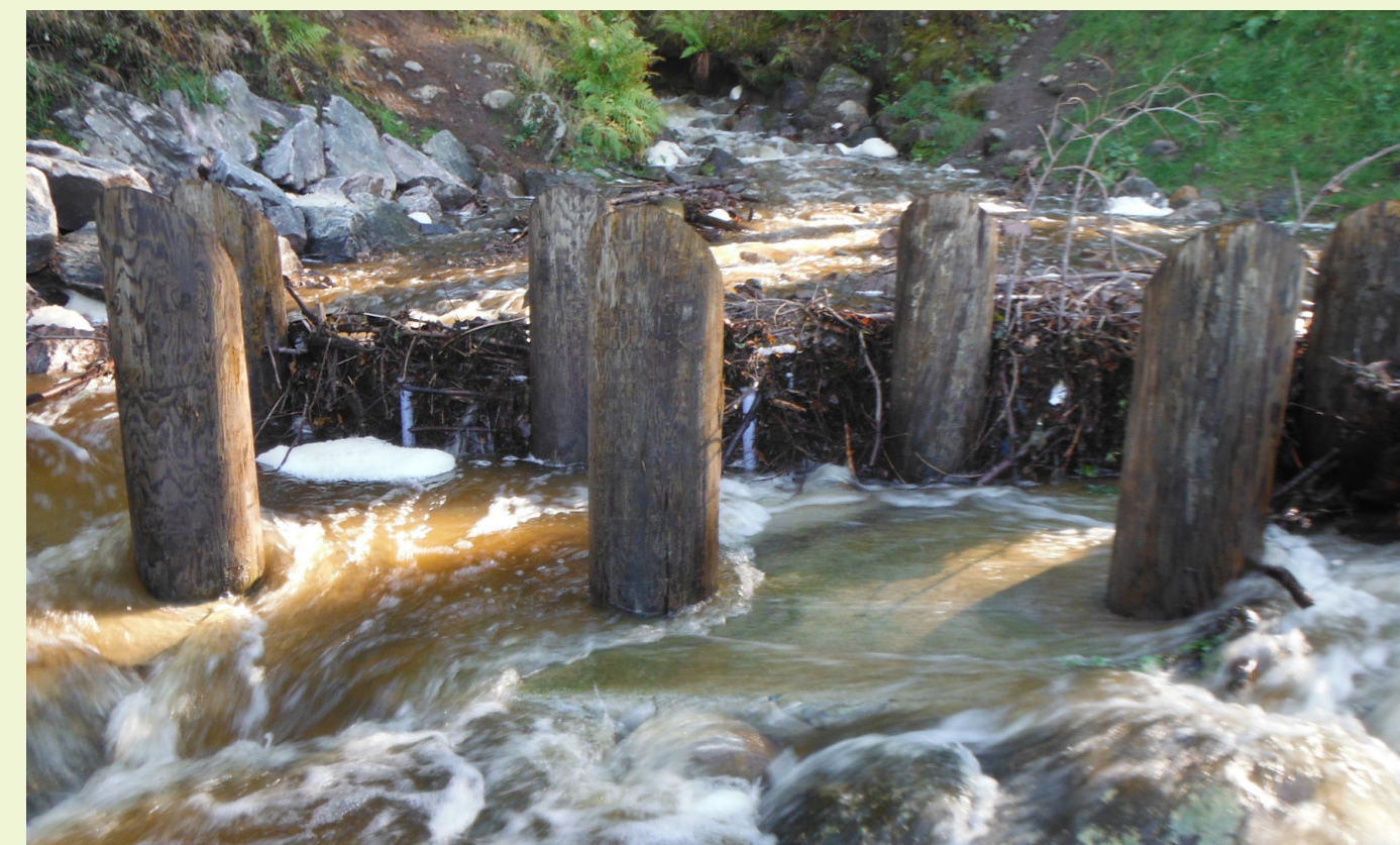
Debris caught on the screen during the 2014 floods may have blocked downstream culverts and caused flooding.
