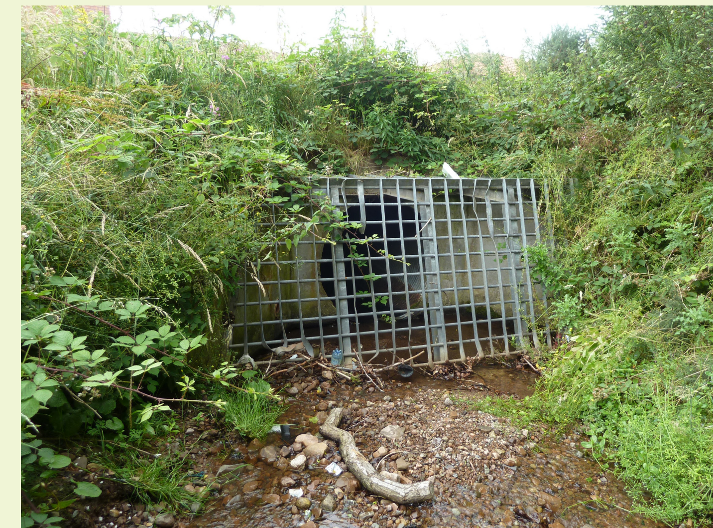
Before: debris screen at Culloden Centre, prone to blockage.
