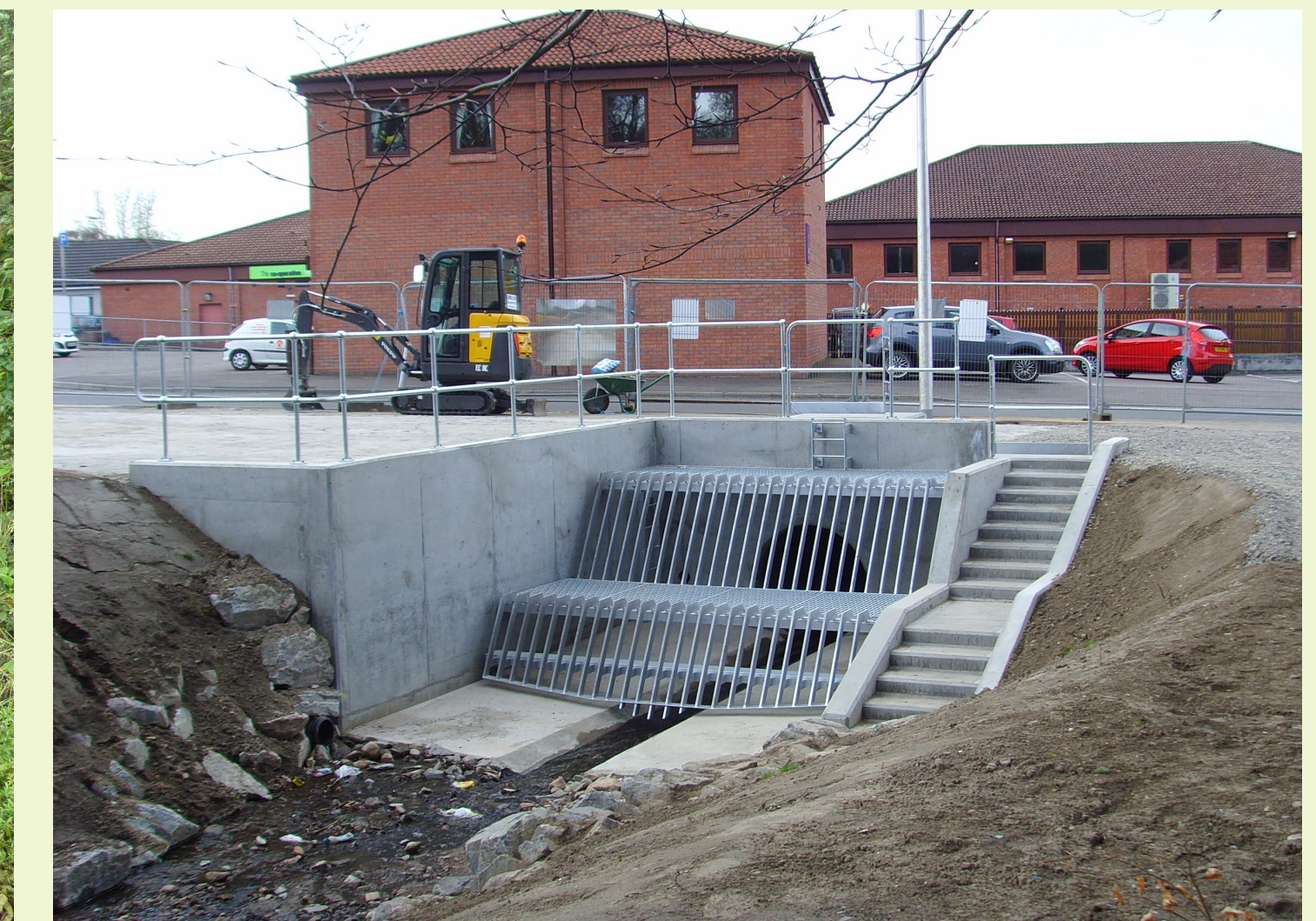
After: new debris screen designed to be resistant to blockage and allow some sediment to pass through the culvert.
