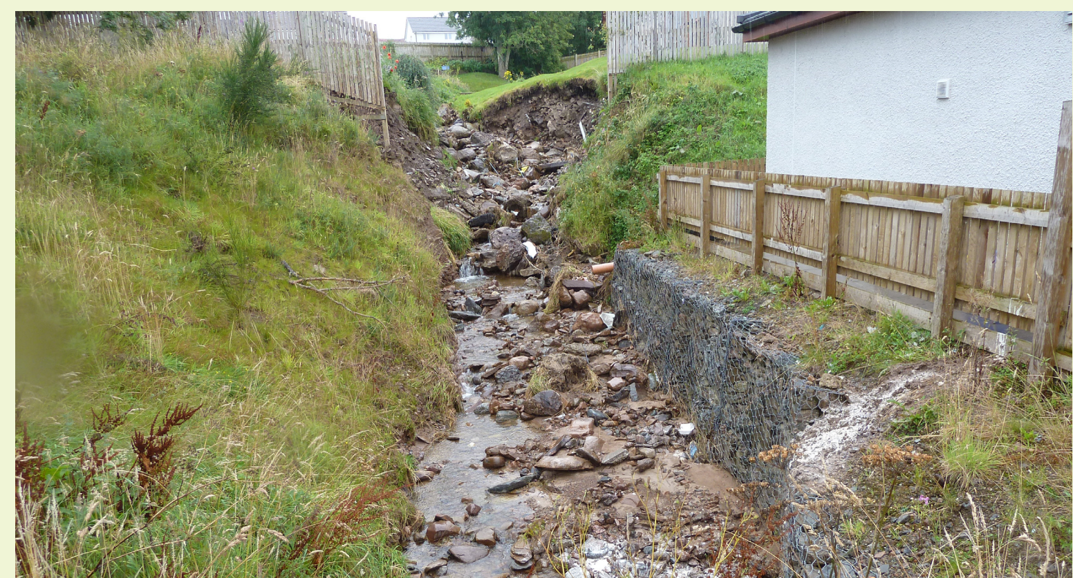
Before: Uncontrolled channel erosion during the 2011 floods increasing the risk of downstream blockage.
