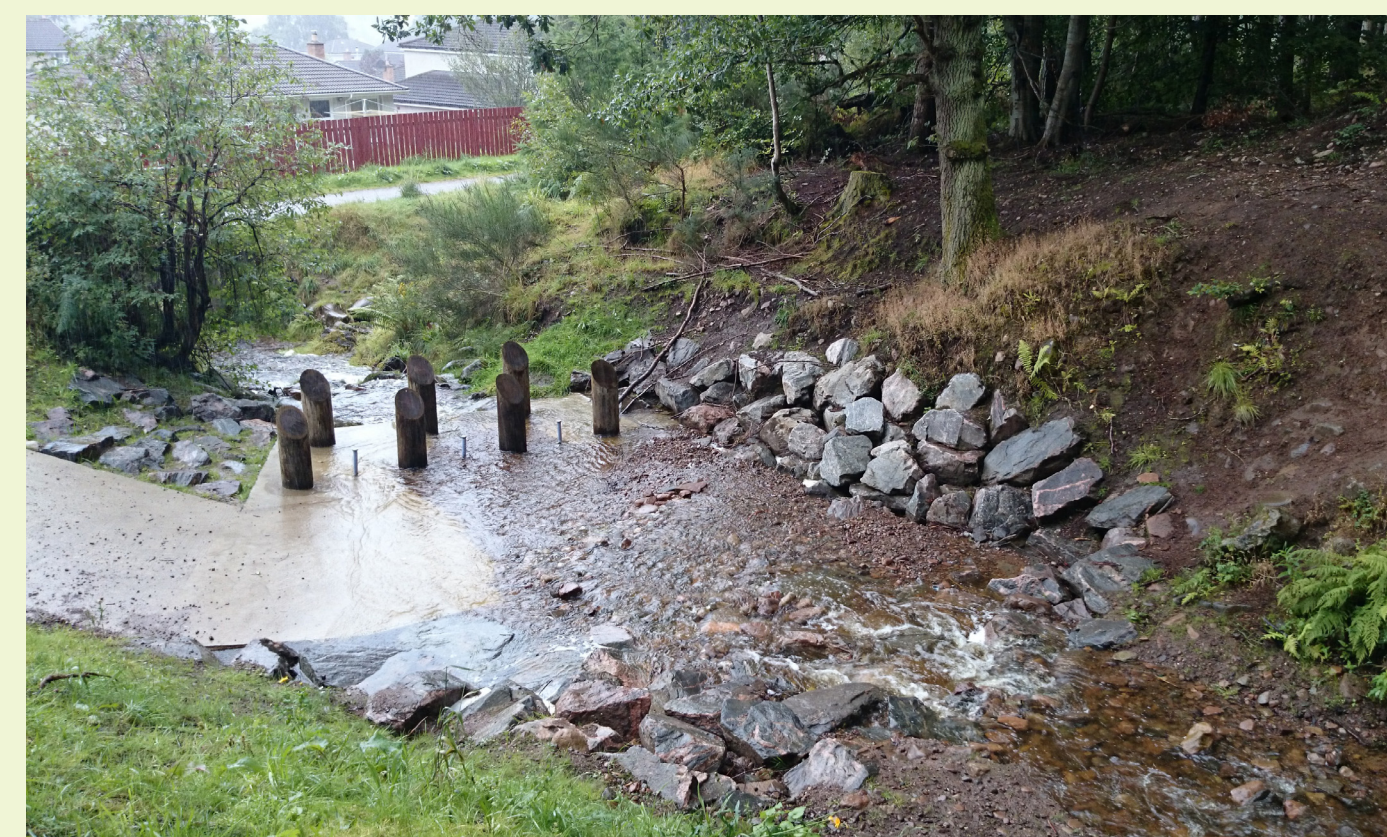
After: New coarse debris screen allows the sustainable movement of sediments, but retains larger material and debris that are likely to block structures.
