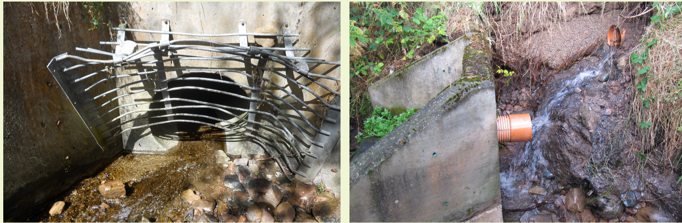
Channels routed underground through culverts are dangerous and prone to blockage and damage. Collapsed headwall
