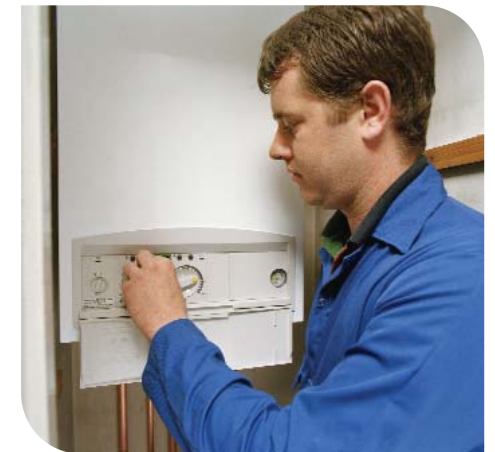
An example of a typical boiler
