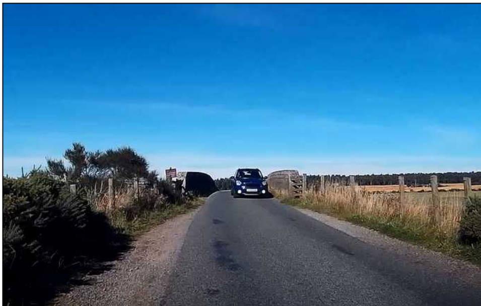
Photo D12 – C1163 Delnies Road facing west at railway bridge crossing (demonstrating space for only one vehicle on bridge)
