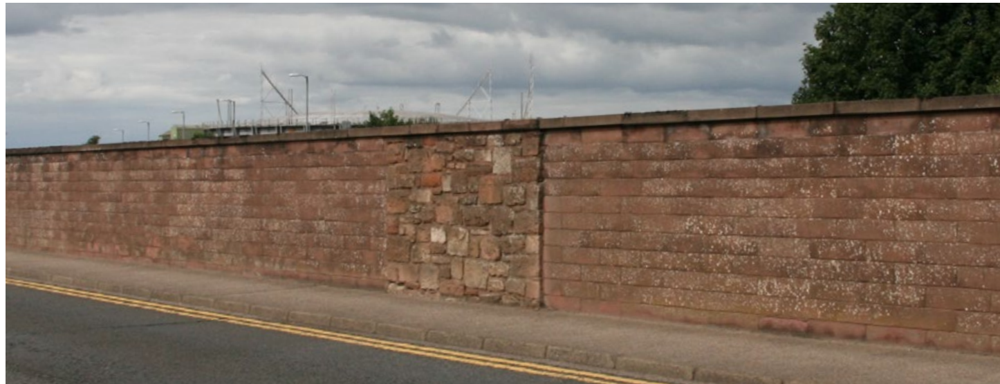
Preferred detail: random rubble stone wall, bought to courses with a heavy plain cope. Alternative detail: stone effect block-work with a heavy plain cope. This photo demonstrates clearly how stone weathers and improves with age whilst blockwork simply fades.
