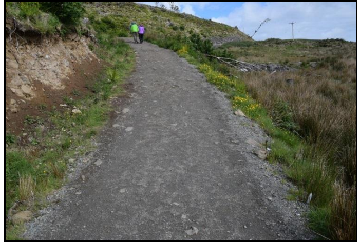
Upgraded path showing slight surface wear
