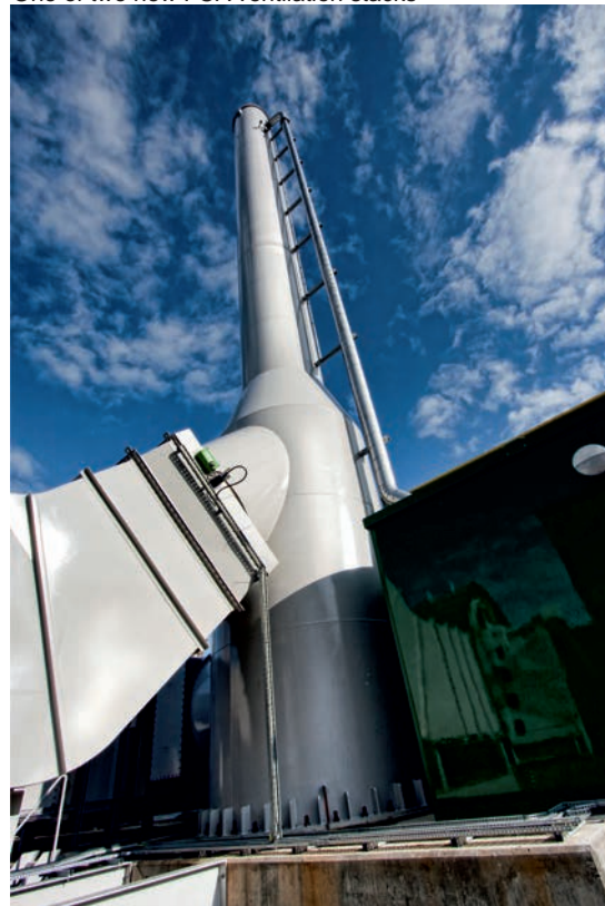
One of two new FCA ventilation stacks
