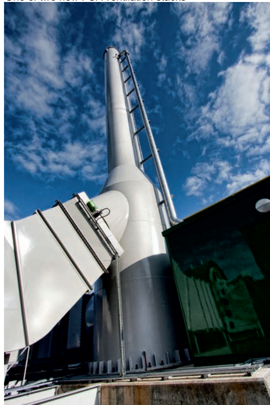
One of two new FCA ventilation stacks
