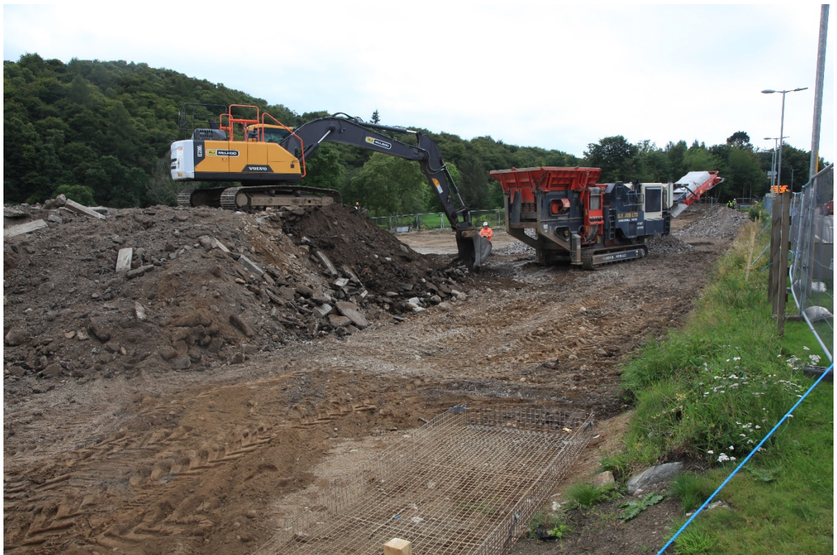
Loading the Crusher with demolished material from the former Torvean Golf Clubhouse
