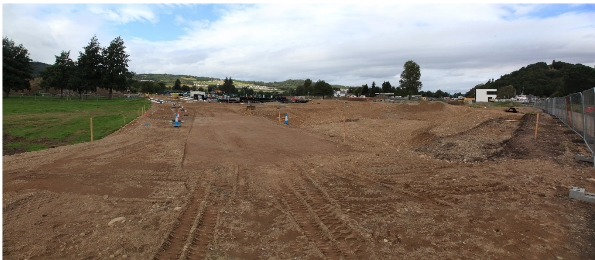
Drainage installation on the new canal access with the new Control Building in the background
