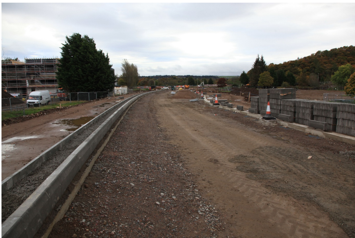
Installing drainage and kerbs and footpaths on the new General Booth Road
