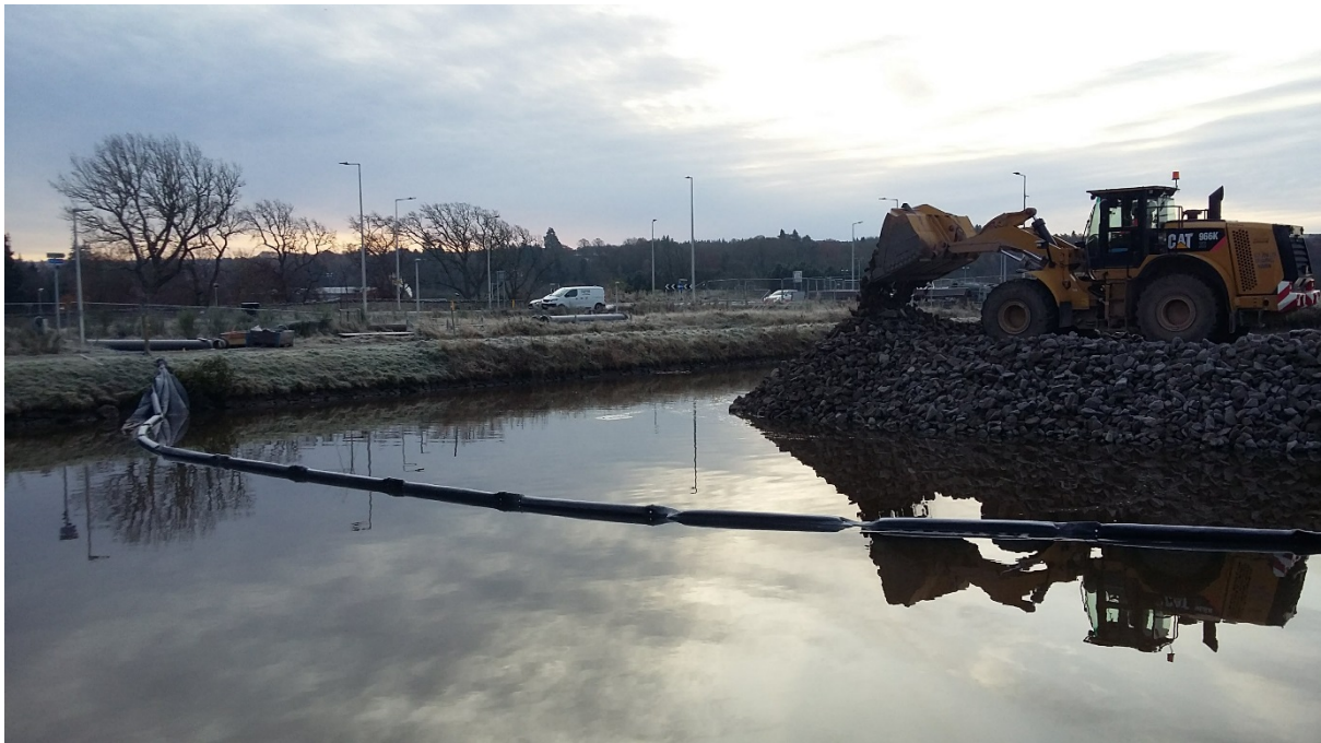
Installing Rock Dam across the canal with wheeled shovel – Silt Curtain in place
