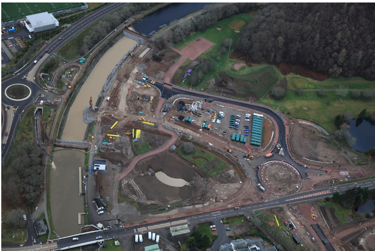
Aerial photo of the site from the North – dams installed and piling rig working on West abutment
