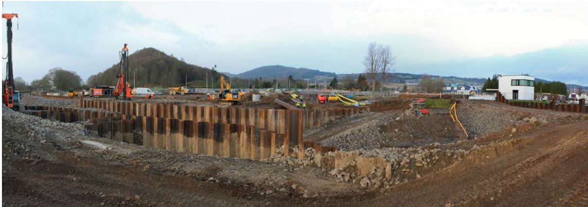
Piling rigs on the East & West abutment, dam and new control tower to the right of the frame
