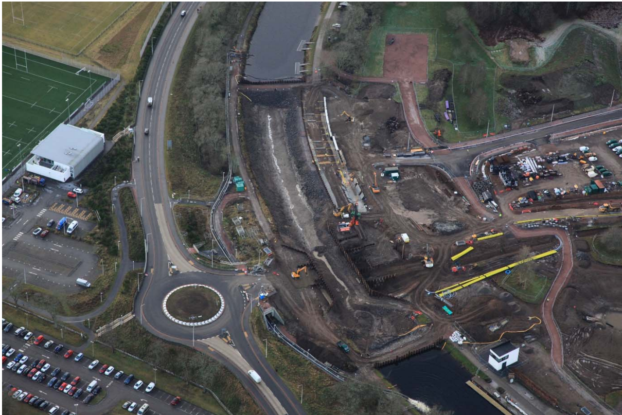
Dewatered section of the canal with piling rig on West abutment and wharf anchor wall progressing
