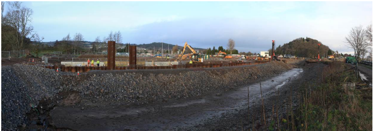
Dewatered section of the canal with the wharf piles and piling on the East & West abutment
