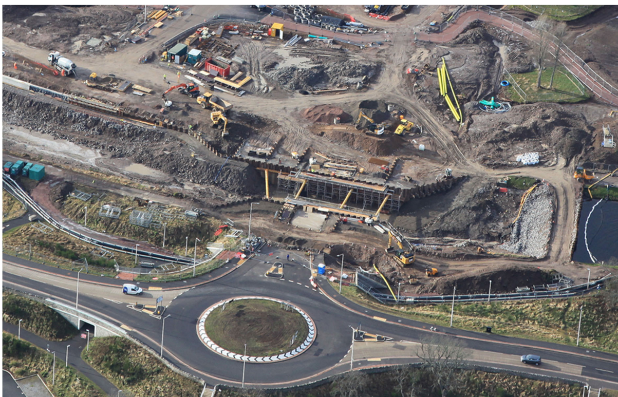
Works progressing on the bridge capping beams on either side of the dewatered canal
