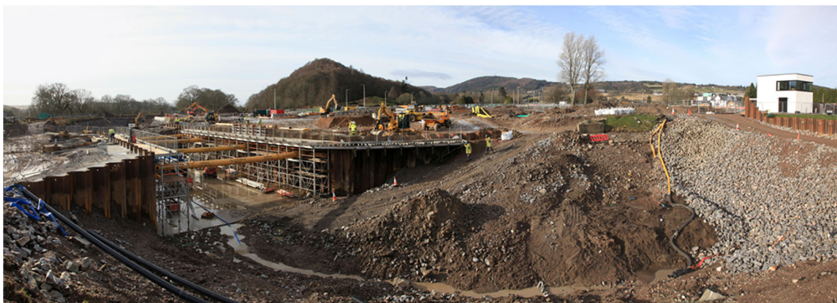
Falsework and propping to allow capping beam construction on the bridge abutments – canal dewatered
