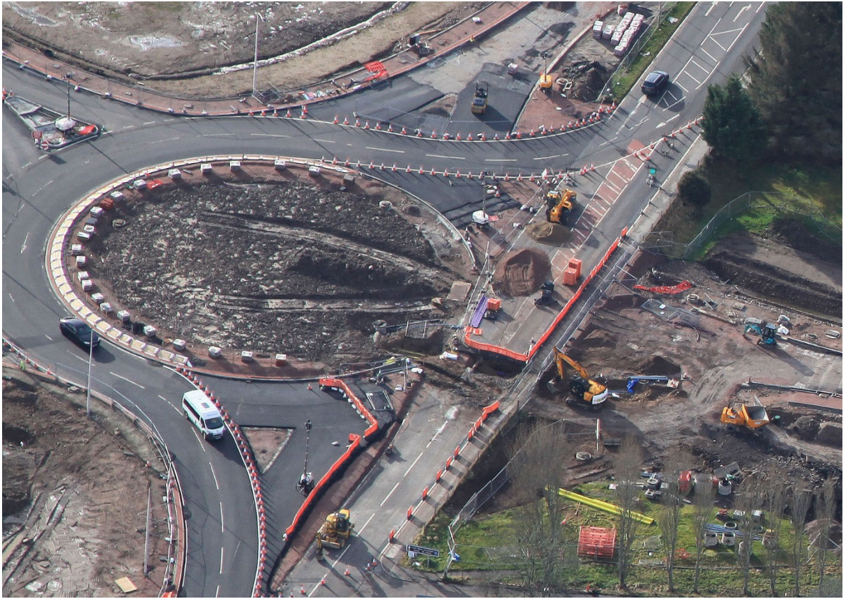
Diversion on the A82 to facilitate the installation of deep drainage and services to the North of the Roundabout
