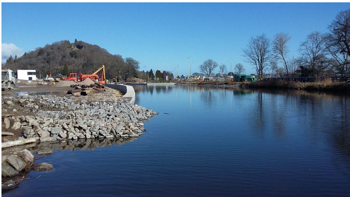
Looking North with the South dam removed and the capping beams on either side of the canal
