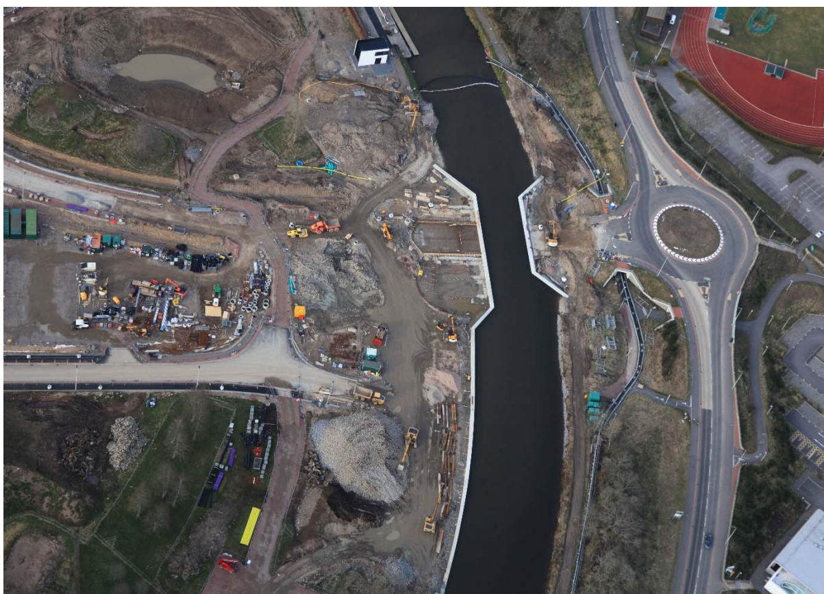
Picture from the South with the canal almost open – silt curtain still to be removed. The works on the concrete apron the bridge can be seen on the left of the canal.
