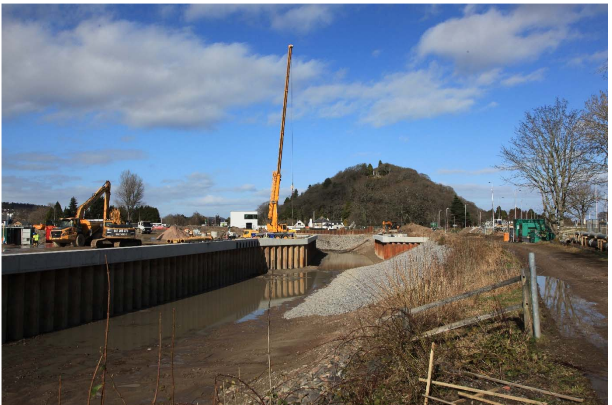
Looking North with the completed works in the canal, wharf, abutments, stone pitching and dam in the foreground
