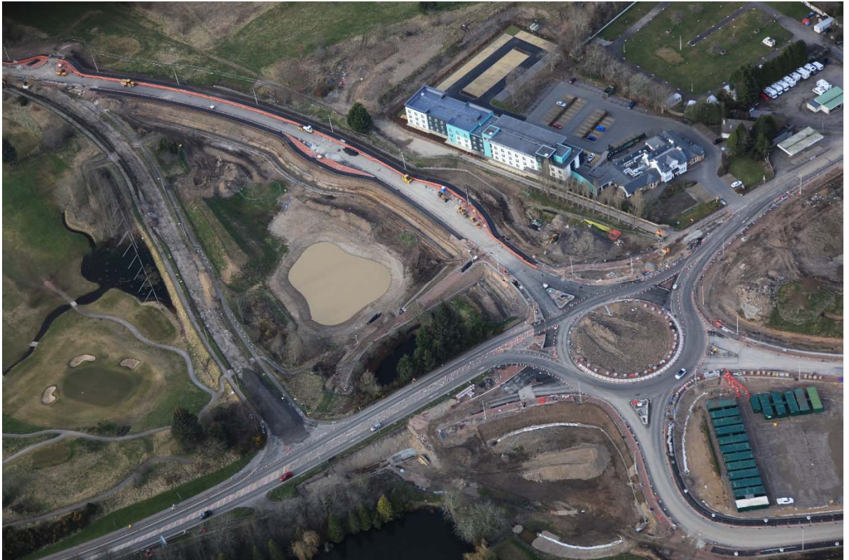
Surfacing Completed to the North of the roundabout to facilitate the removal of the HGV diversion and the closure of General Booth Road.
