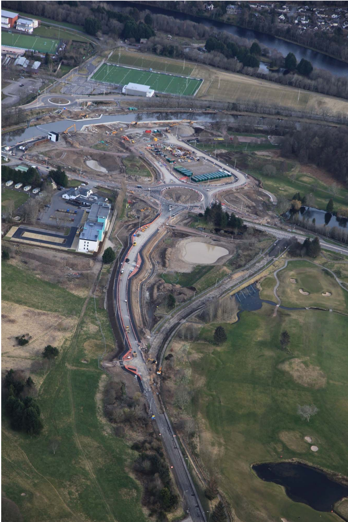
A view of the site from the North. This shows the canal refilled and the existing section of General Booth Road with the surfacing removed.
