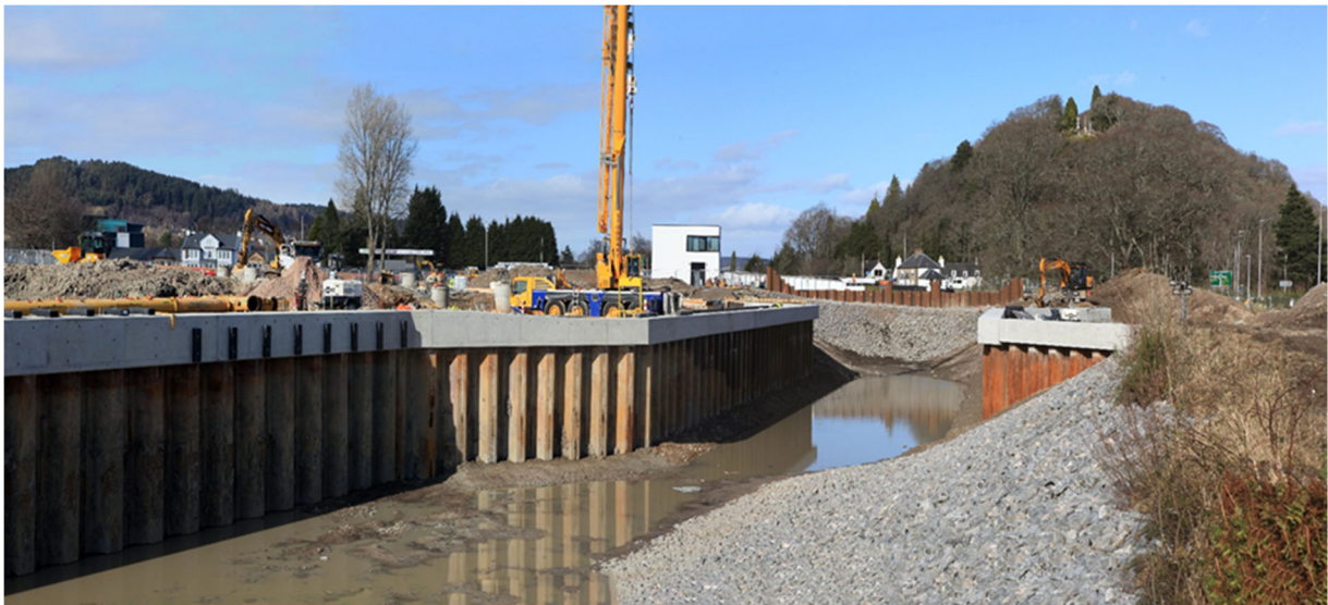
Re-watering of the canal in March following completion of concrete capping beams
