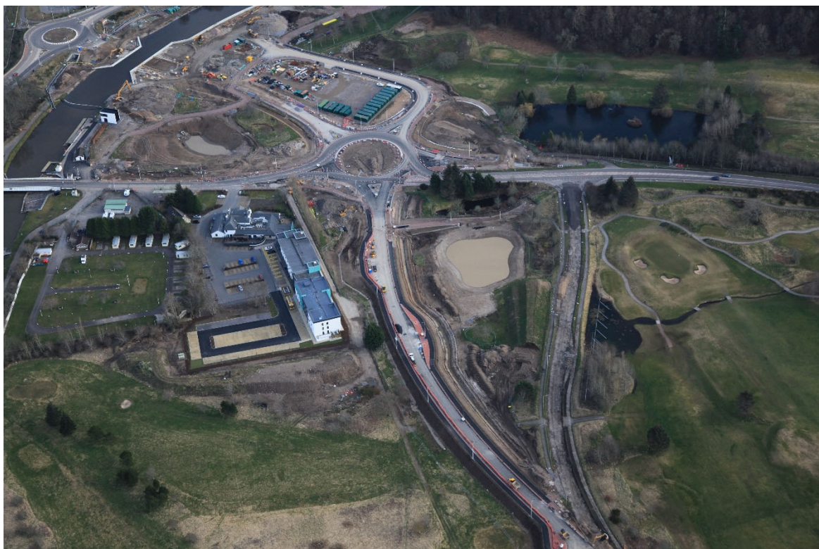
Aerial photo of the site from the North with the old General Booth Road planned, concrete capping beam complete and canal re-watered
