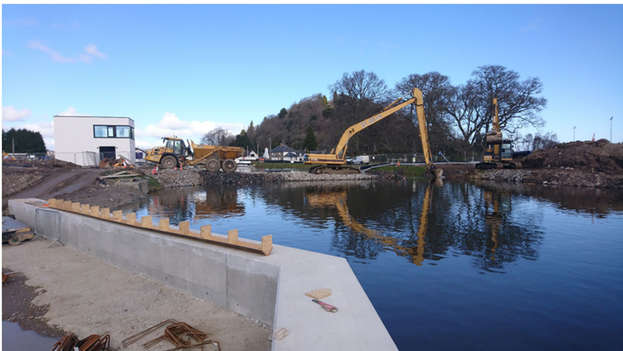
Removal of stone dams from the canal using long reach excavator with GPS machine control
