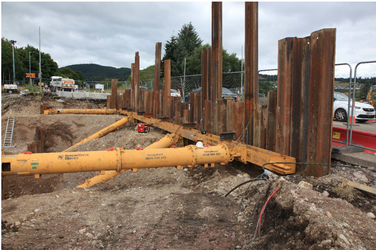
Sheet piles and bracing installed adjacent to the A82 to facilitate the installation of the underpass
