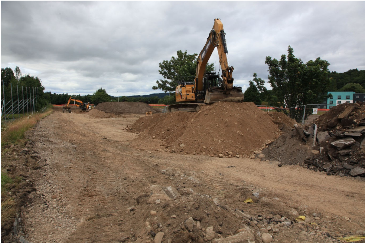
Excavation works on the old General Booth Road to make way for ponds and golf tees
