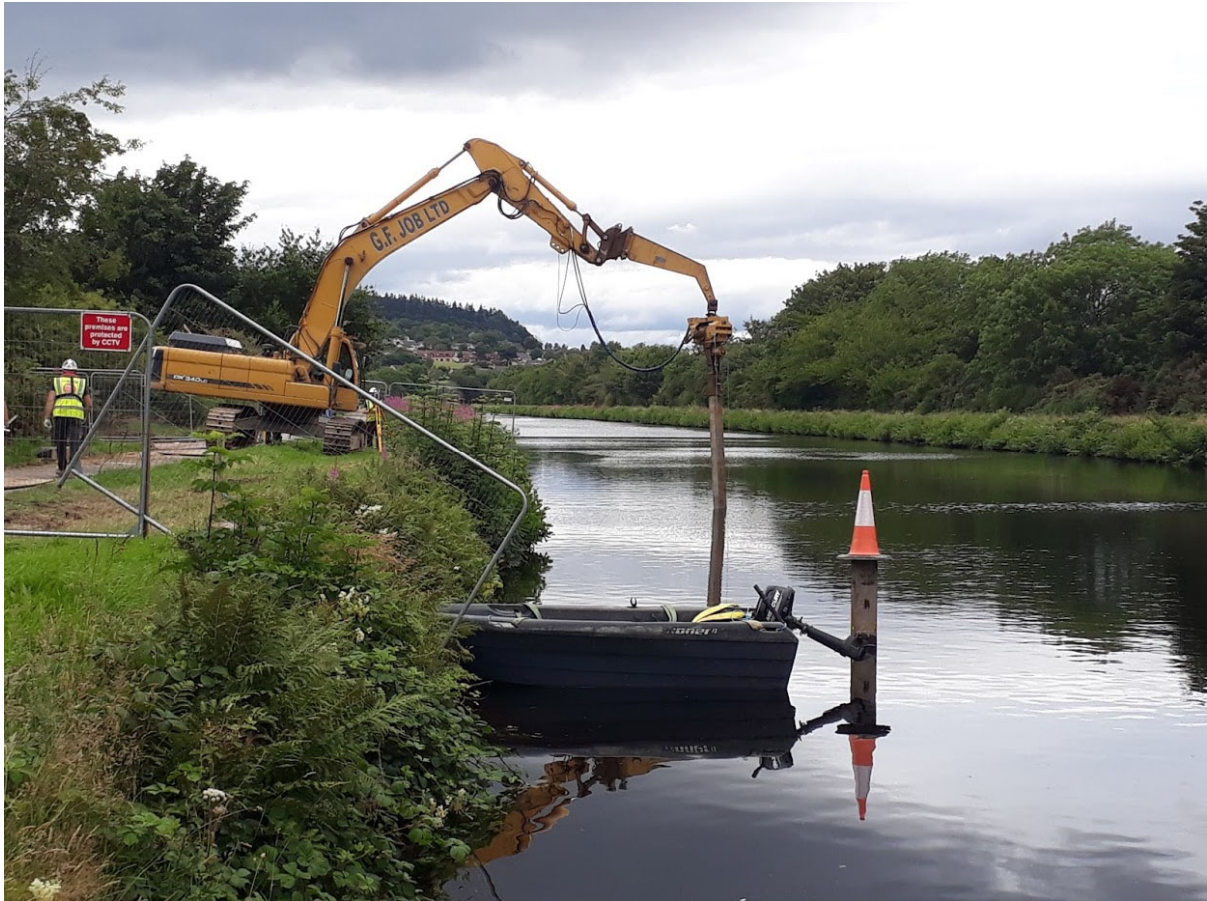
Excavator installing timber piles in the canal for the new timber jetty
