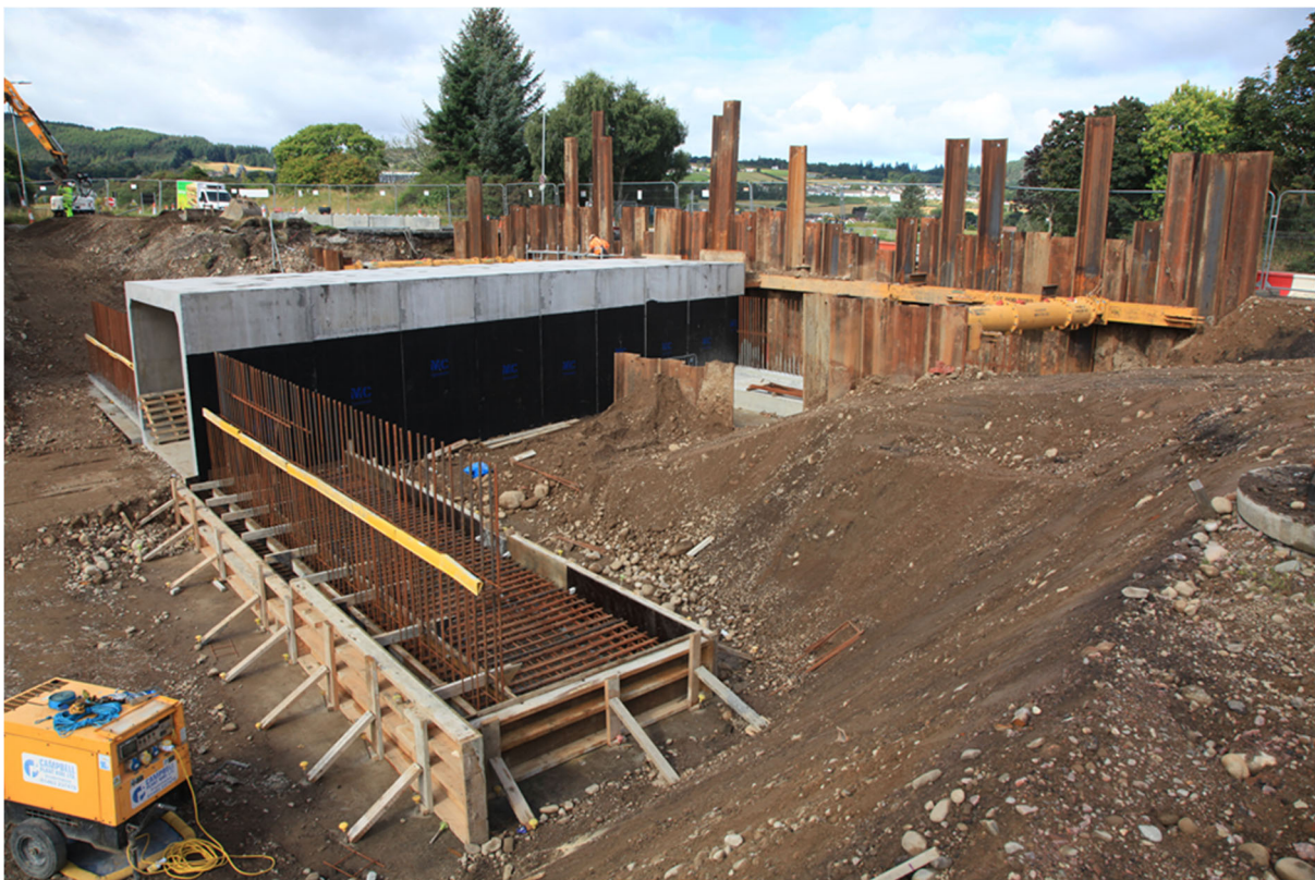
Box Culvert Underpass installed and works progressing on the concrete wing walls
