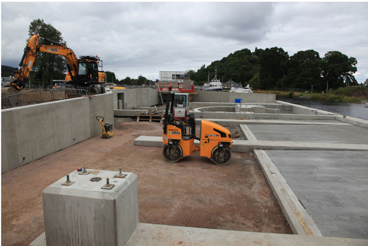
Preparing the concrete slabs and aprons for the new swing bridge, plant room blockwork progressing
