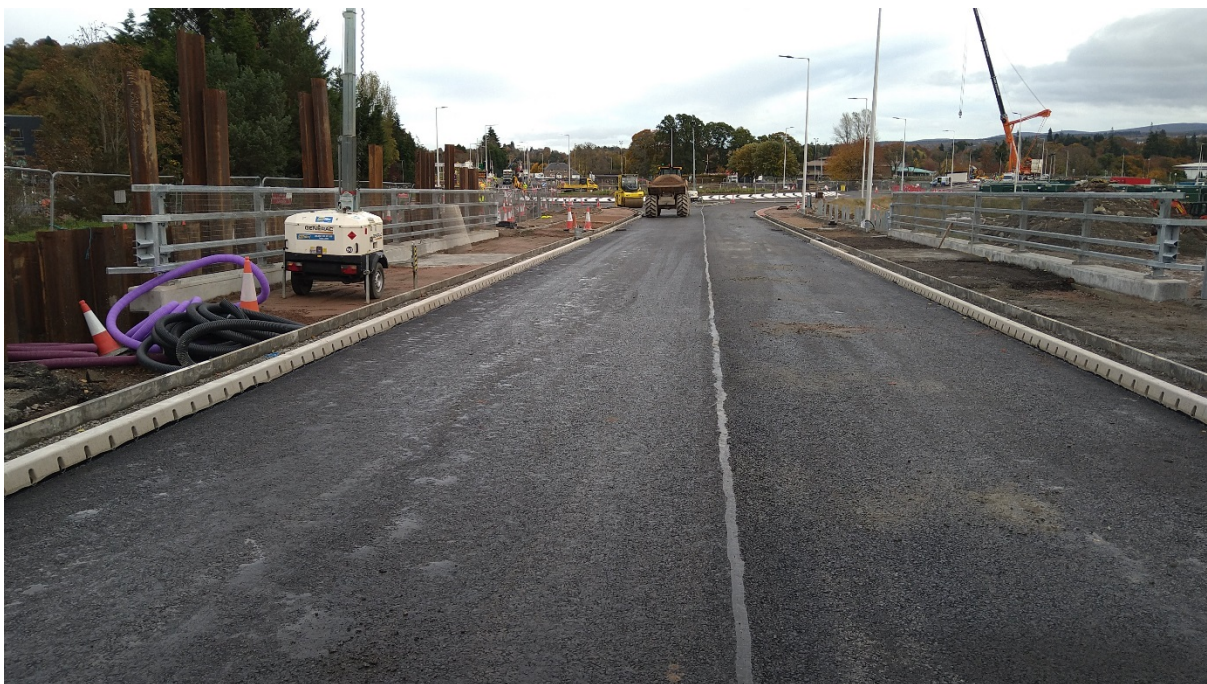
Surfacing over the new Underpass on the A82 with the parapets and safety fencing in the process of being erected
