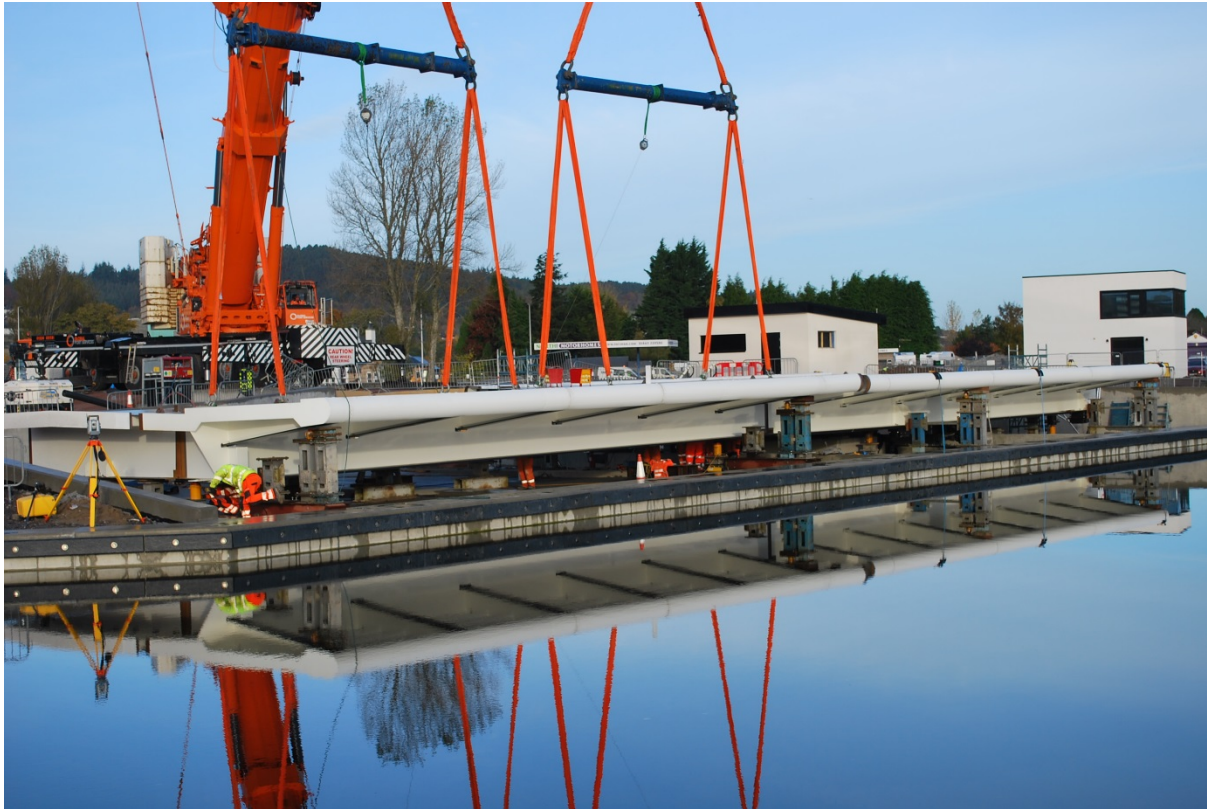
The bridge in position with the temporary supports and jacks supporting the bridge sections
