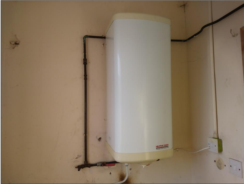
Photograph 9 – Water Heater (Utility Room)
