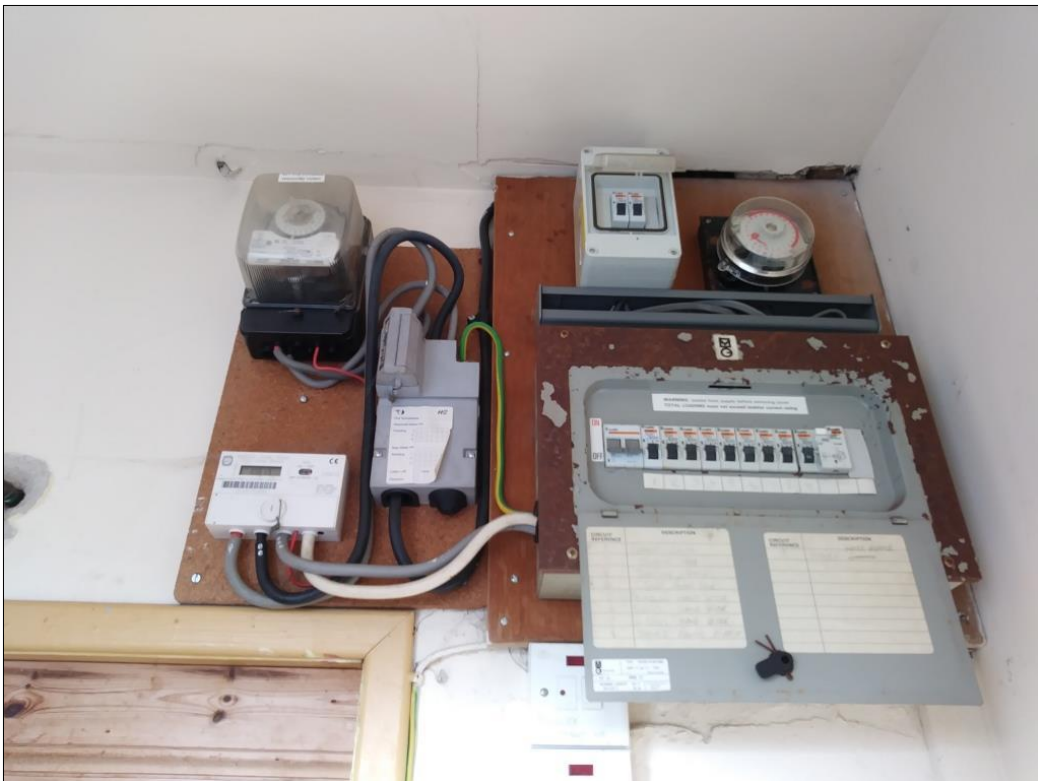
Photograph 8 – Electricity Distribution Board & Meter (Utility Room)
