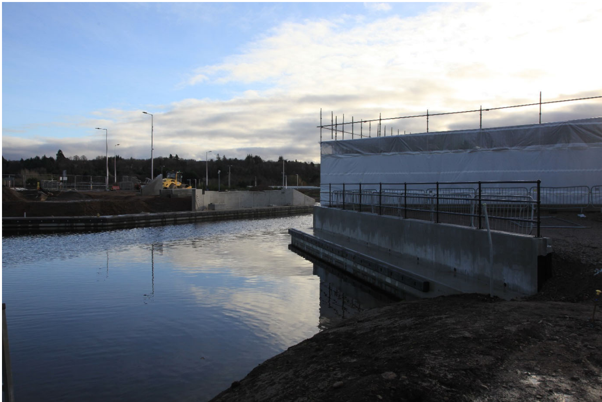
Looking South from the West abutment onto the East abutment wall and the encapsulation over the new swing bridge
