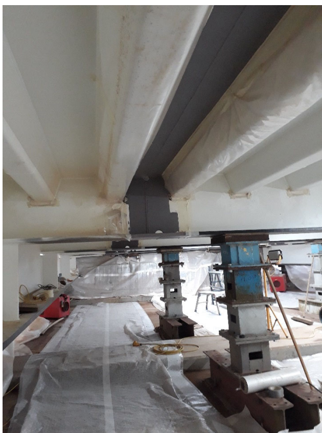
Painting of the welded joints with the temporary propping evident for supporting the bridge
