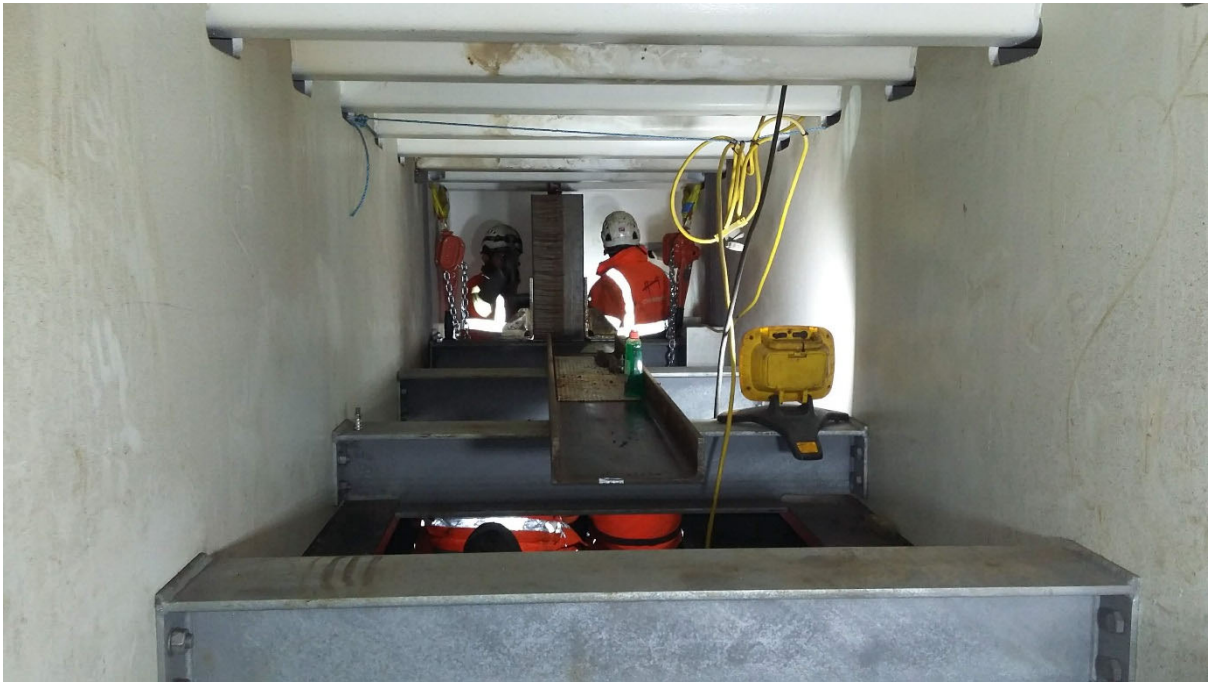
Installation of the steel ballast blocks to the rear of the bridge
