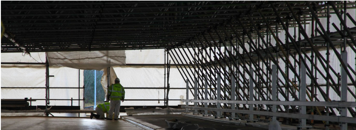
Waterproofing of the bridge deck and the bridge parapets installed along the edge of the footway
