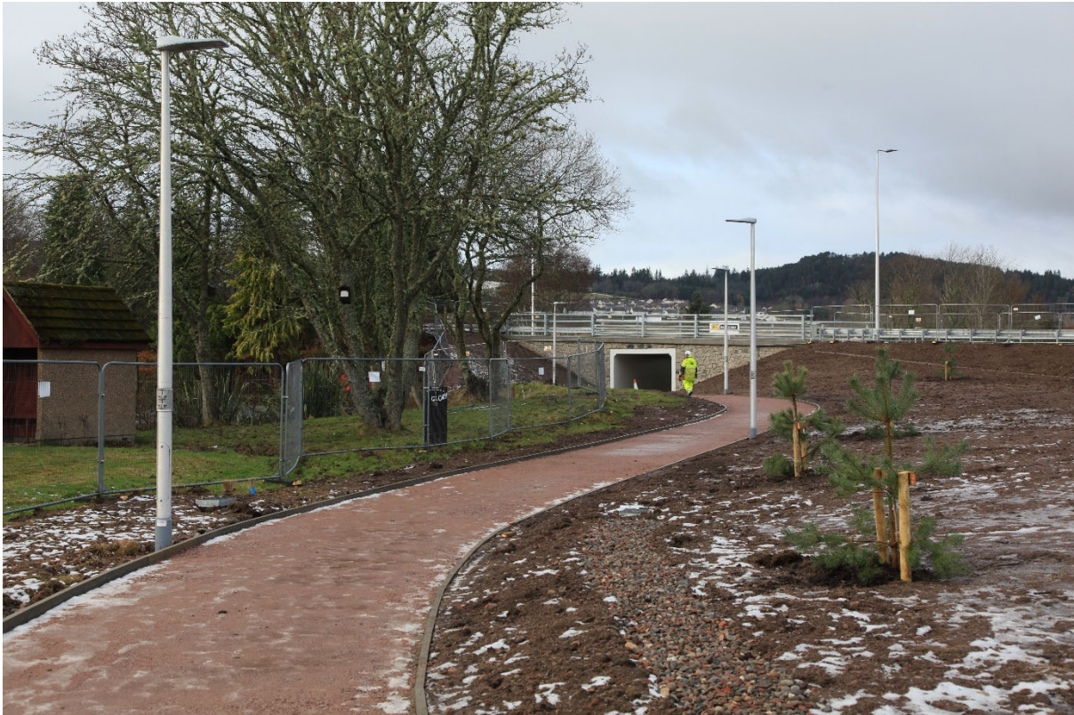
Looking West to the new underpass under the A82 – footpath ready for surfacing
