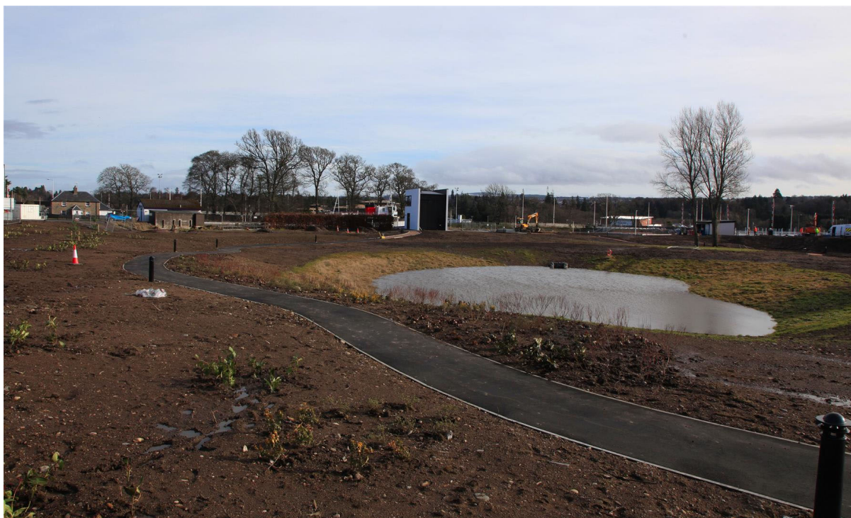
Looking East across the new pond towards the new control building, footpaths and planting
