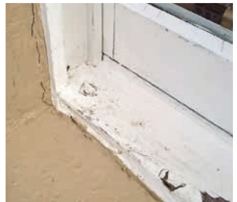
Cracked and peeling paint
