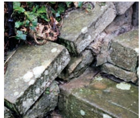
Plant roots damaging stonework
