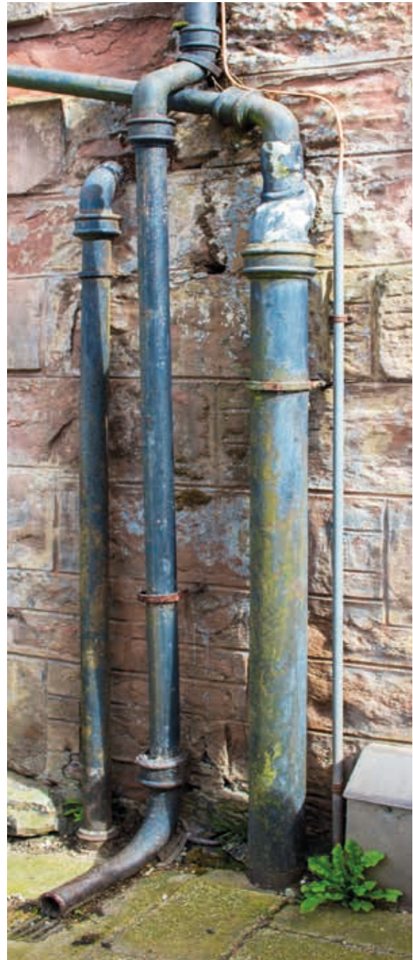
Spaghetti plumbing - changes over the years!
