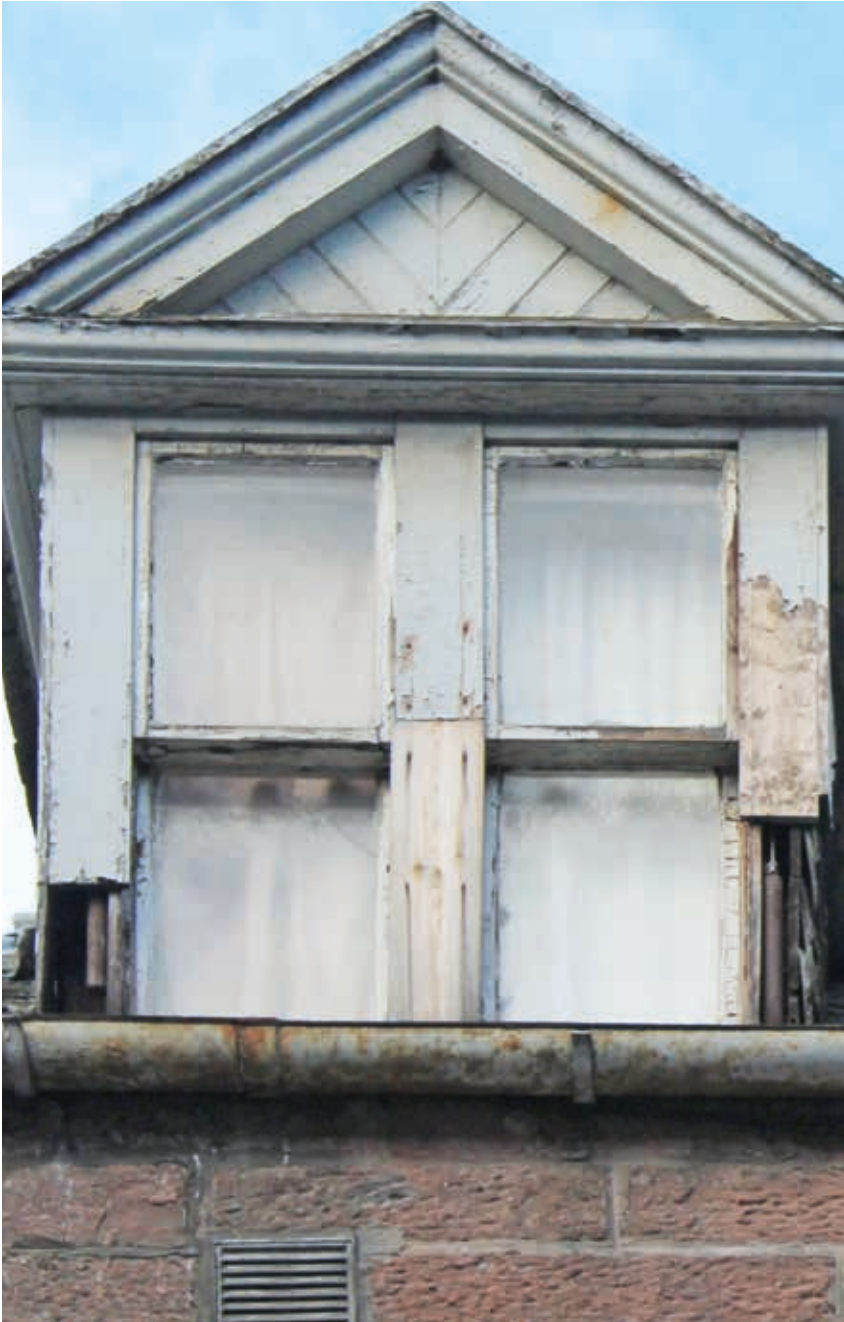
Missing cladding panels
