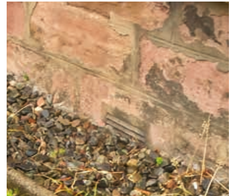
High ground levels blocking ventilation
