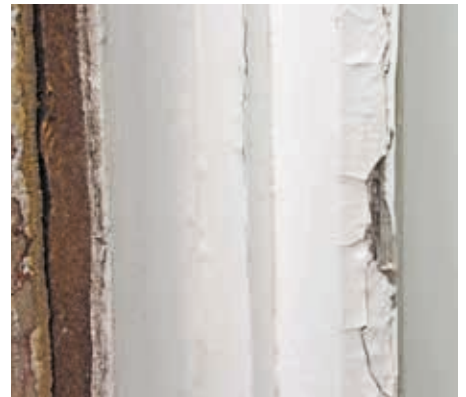
Cracked and missing putty
