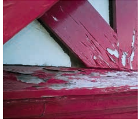
Cracked and peeling paint
