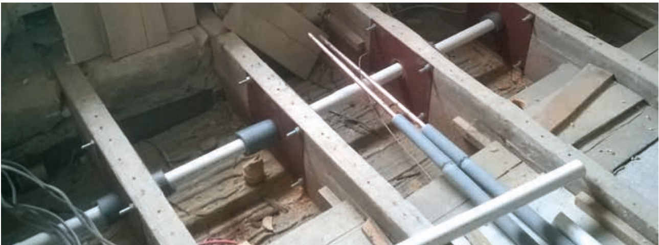
Removal of sound insulation to install services without compromising strength of floor
