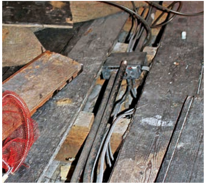
Notching reduces strength of timber
