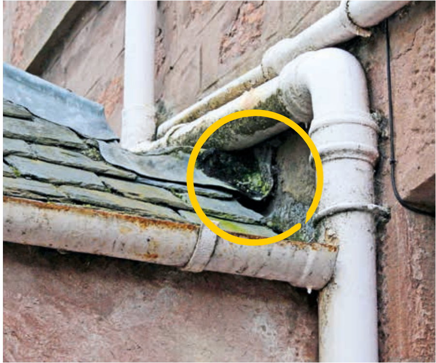
Awkward drainage junctions
