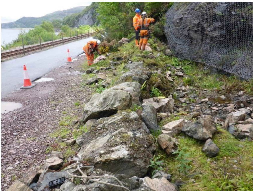
Photo 3: Edge of debris catch pit between toe of slope and road. Recent debris visible on both side of 'bund' formed of boulders sourced from previous scaling works from adjacent rock cuttings.
