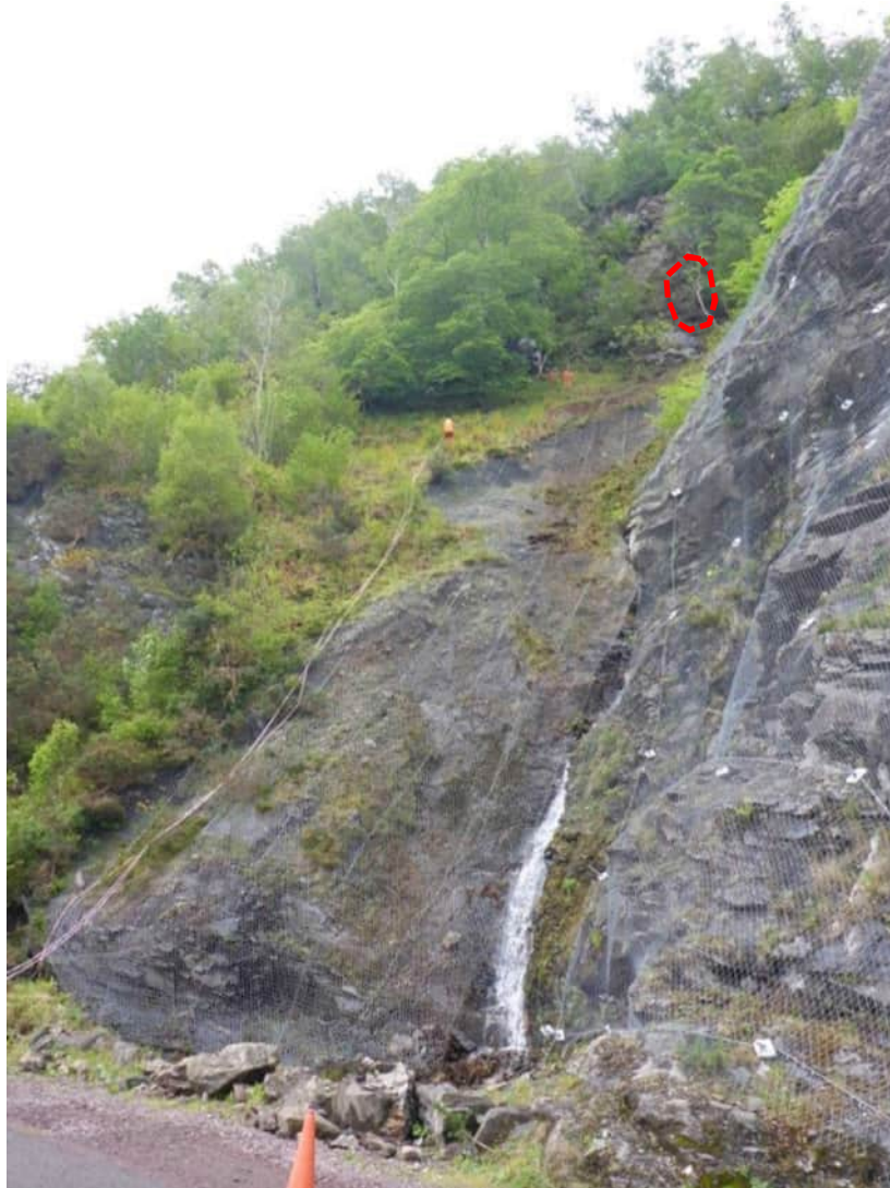
Photo 1: Slope at AA18-AA19 with failure source area circled.
