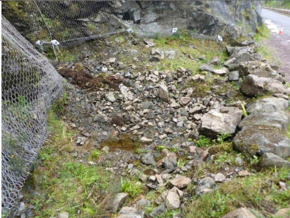
Photo 2: Debris catch pit between toe of slope and road with recent debris accumulation.
