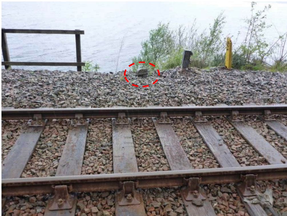
Photo 5: Block located in railway cess on far side of railway. This block is thought to have originated from the recent failure.
