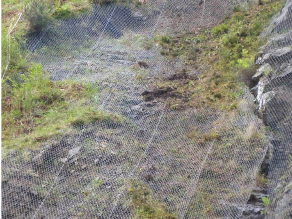
Photo 12: Small tears visible in drape netting system caused by recent failure.
