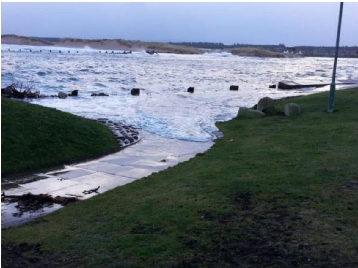
Wave Overtopping in Lossiemouth
