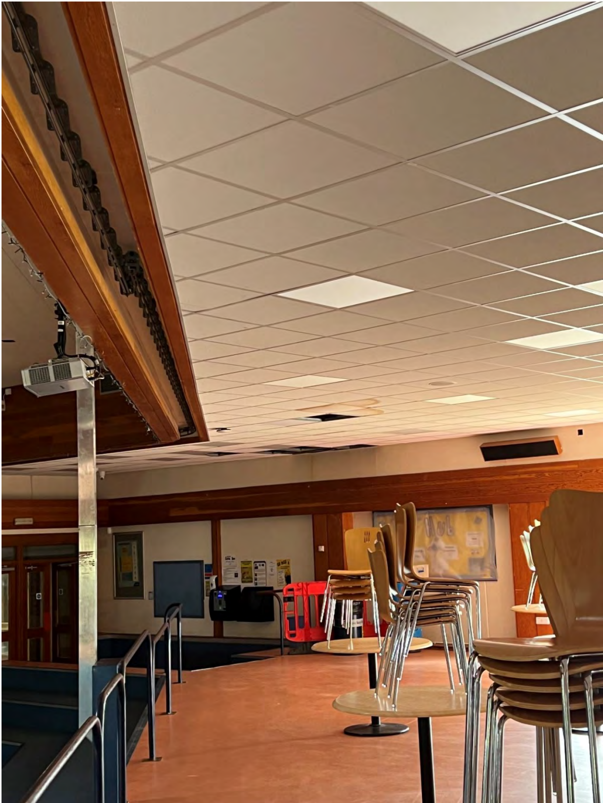
Photo N.17 – Water staining to ceiling however roof construction appears to be profiled metal deck in main hall (Assembly Hall)
