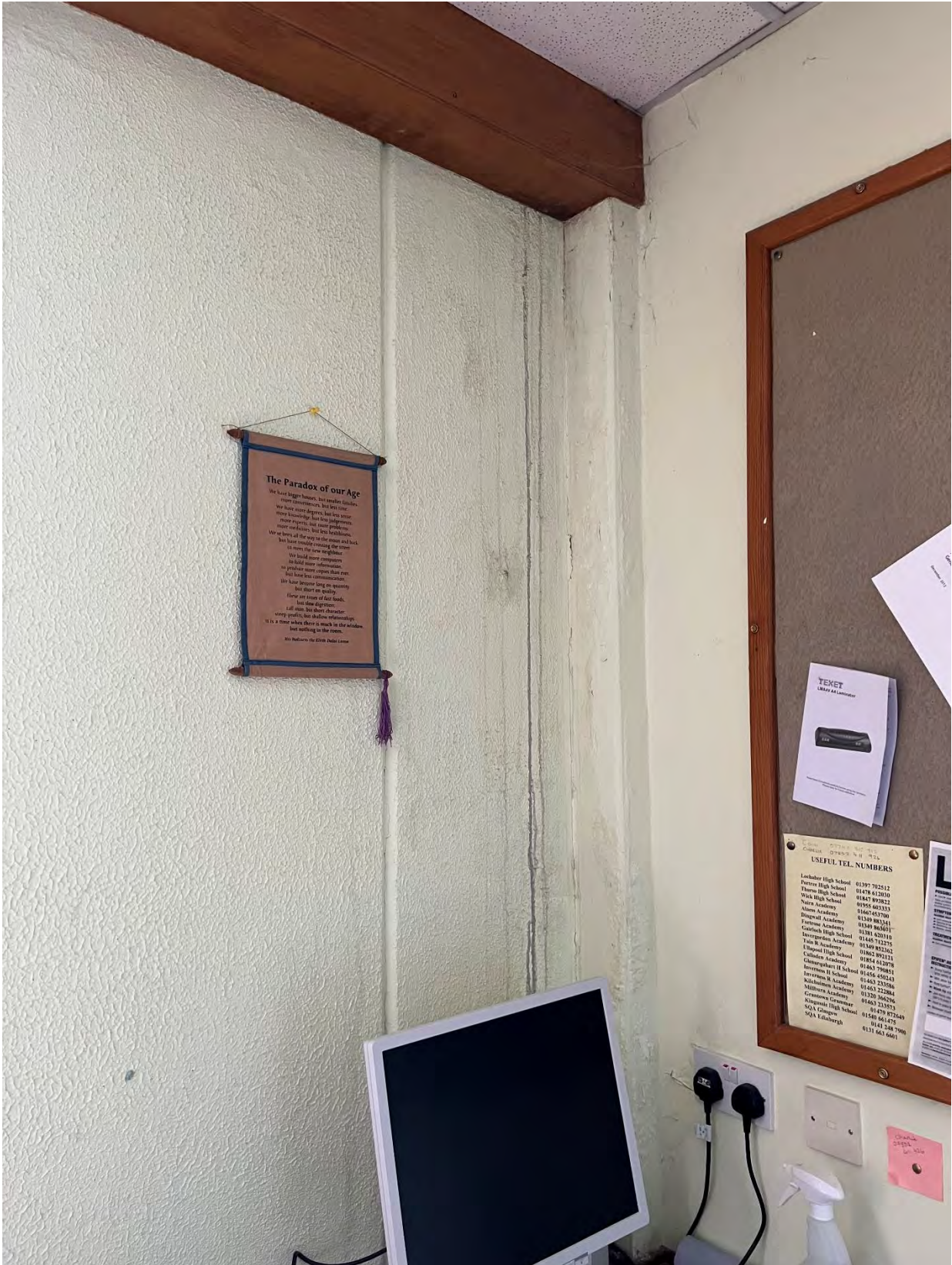
Photo N.10 - Internal view of Siporex Wall panels with water damage (Science Dept)
