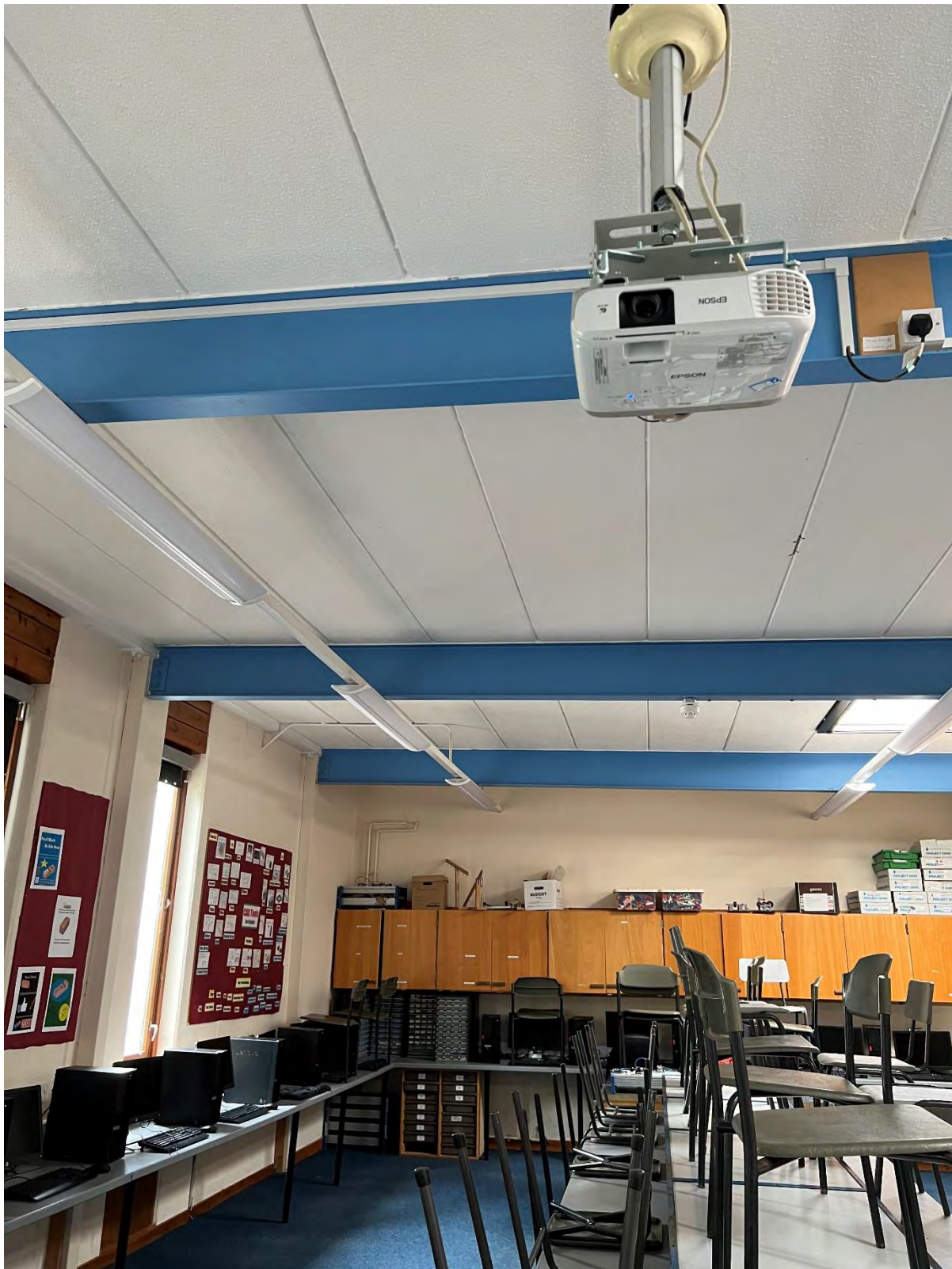
Photo N.5 - Bearing length appears to be less than 75mm throughout (Science Dept)
