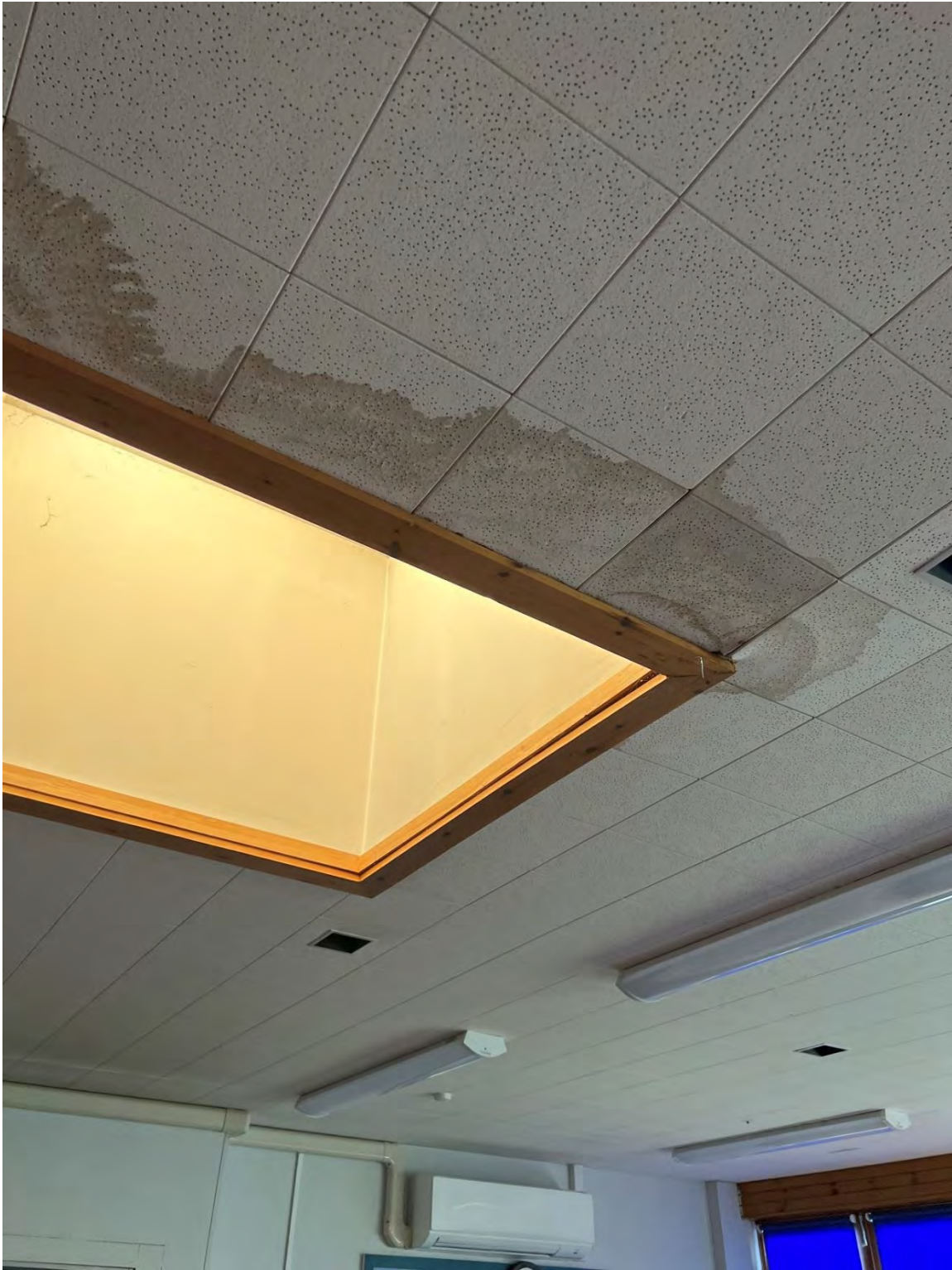
Photo N.14 - Water staining on ceiling tiles indicates potential water ingress (Staff Room)
