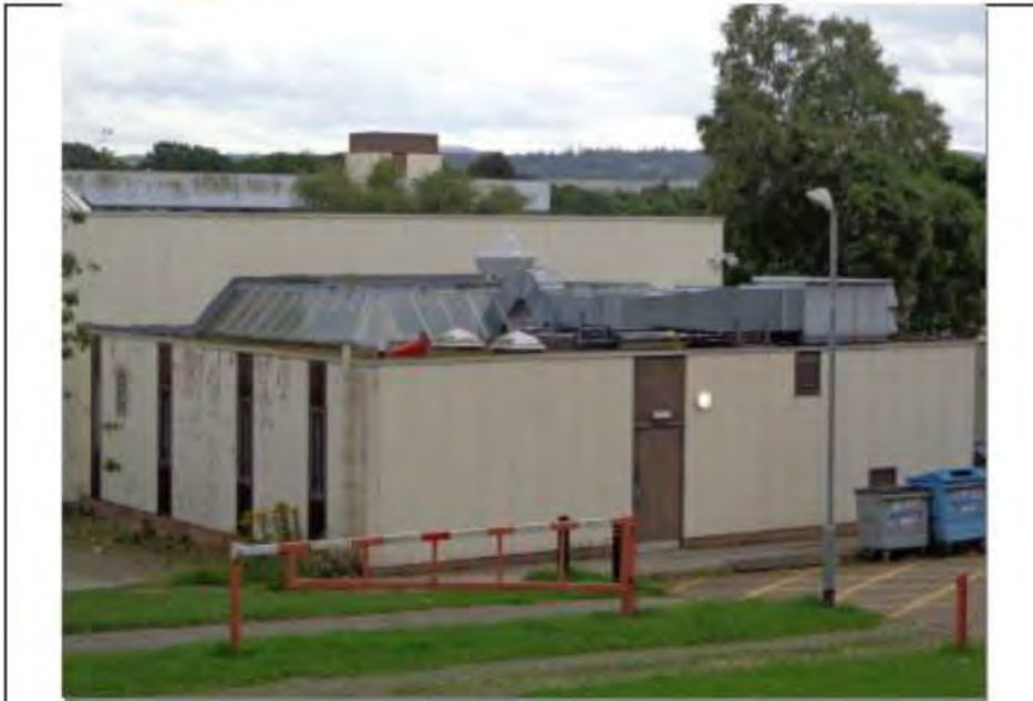
Photo No 5 – Weathering to outside of Siporex wall panels
