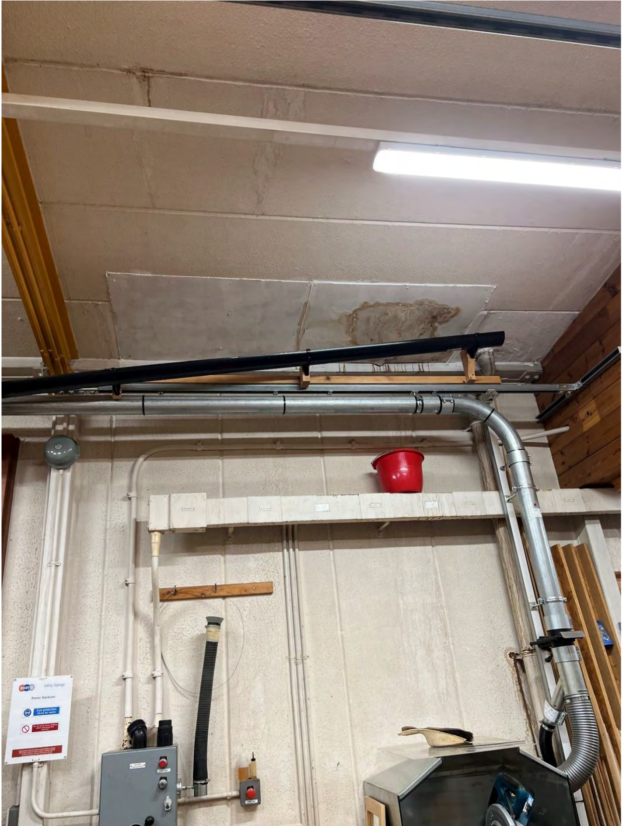
Photo N.3 – Water damage to Siporex panels (Tech Dept)
