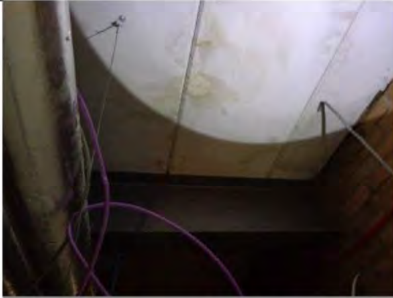
Photo No 3 – Water staining on the underside of panels above a suspended ceiling
