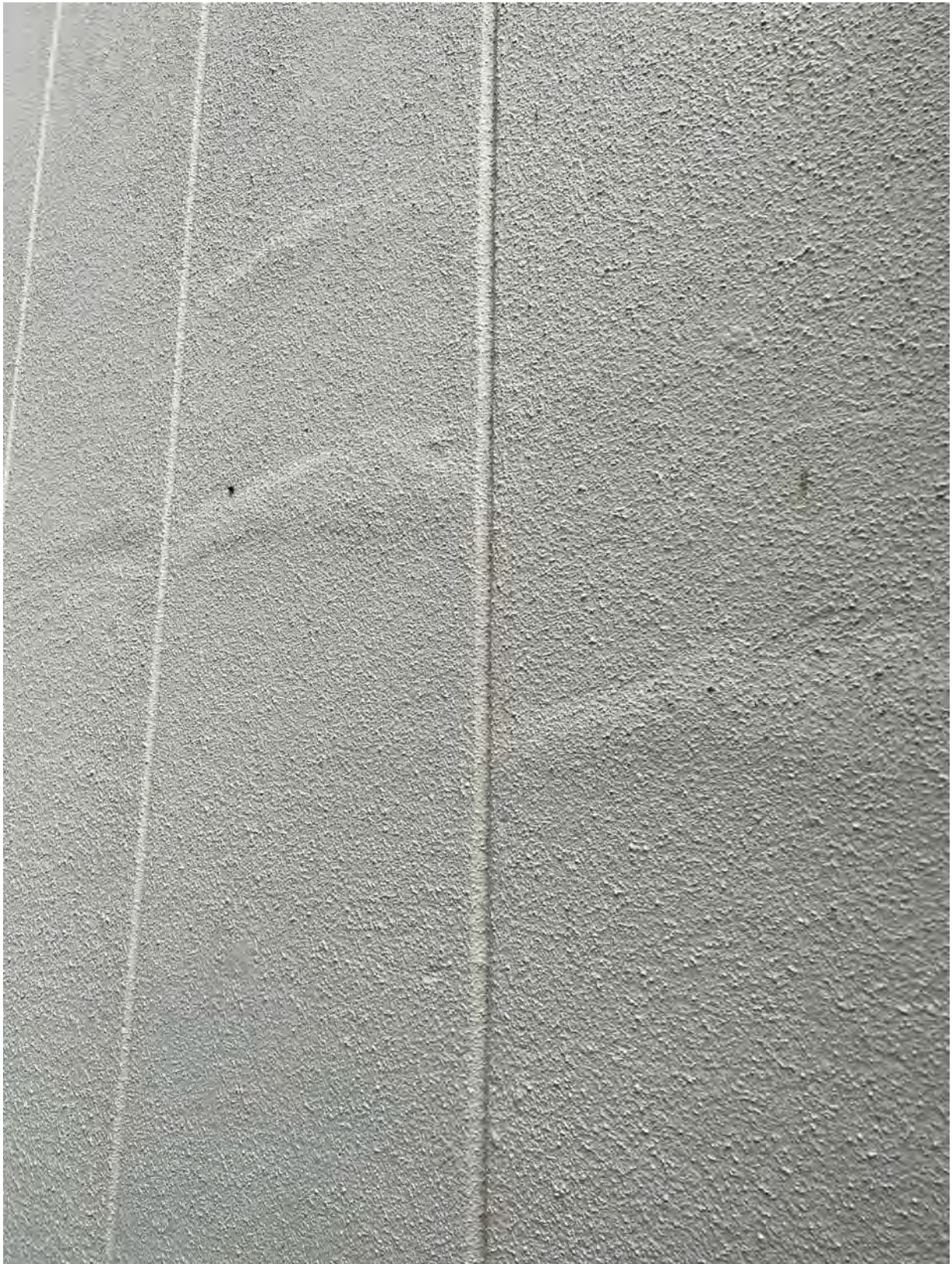
Photo N.9 – Deviations in Siporex Wall panels may indicate water ingress (Art Dept)
