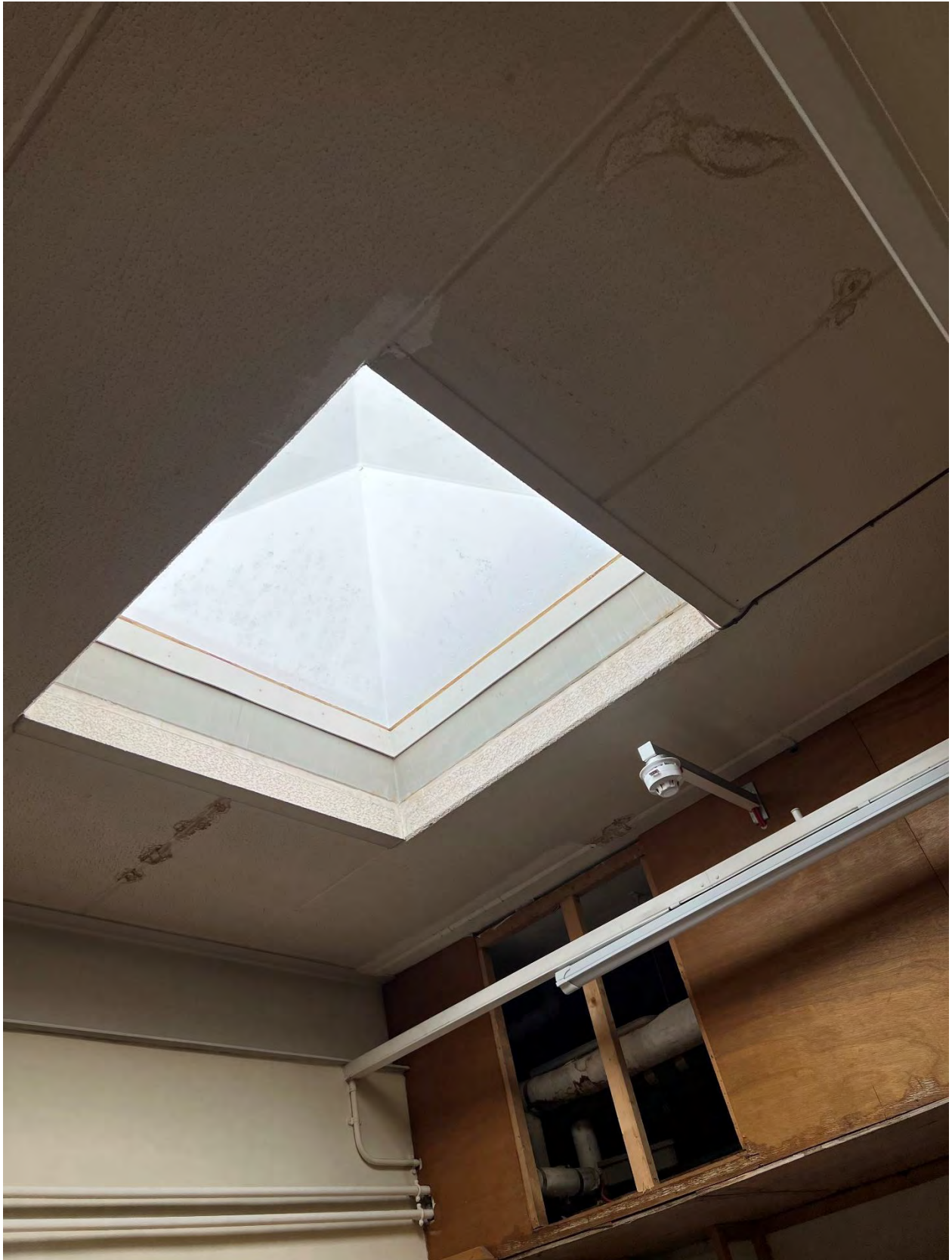
Photo N.7 - Water damage to Siporex panels (Science Dept)
