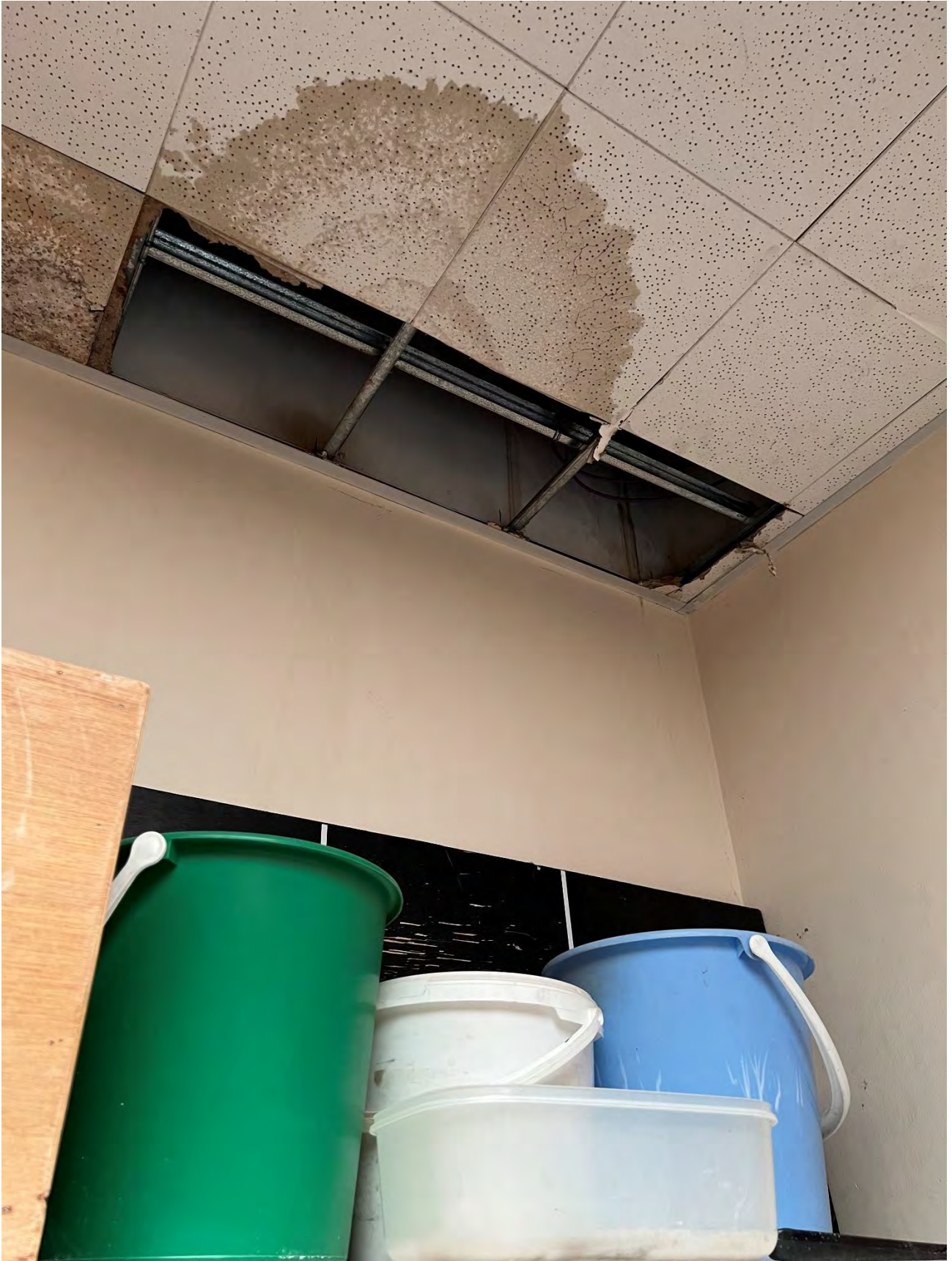
Photo N.15 - Water staining on ceiling tiles indicates potential water ingress (Admin Area)
