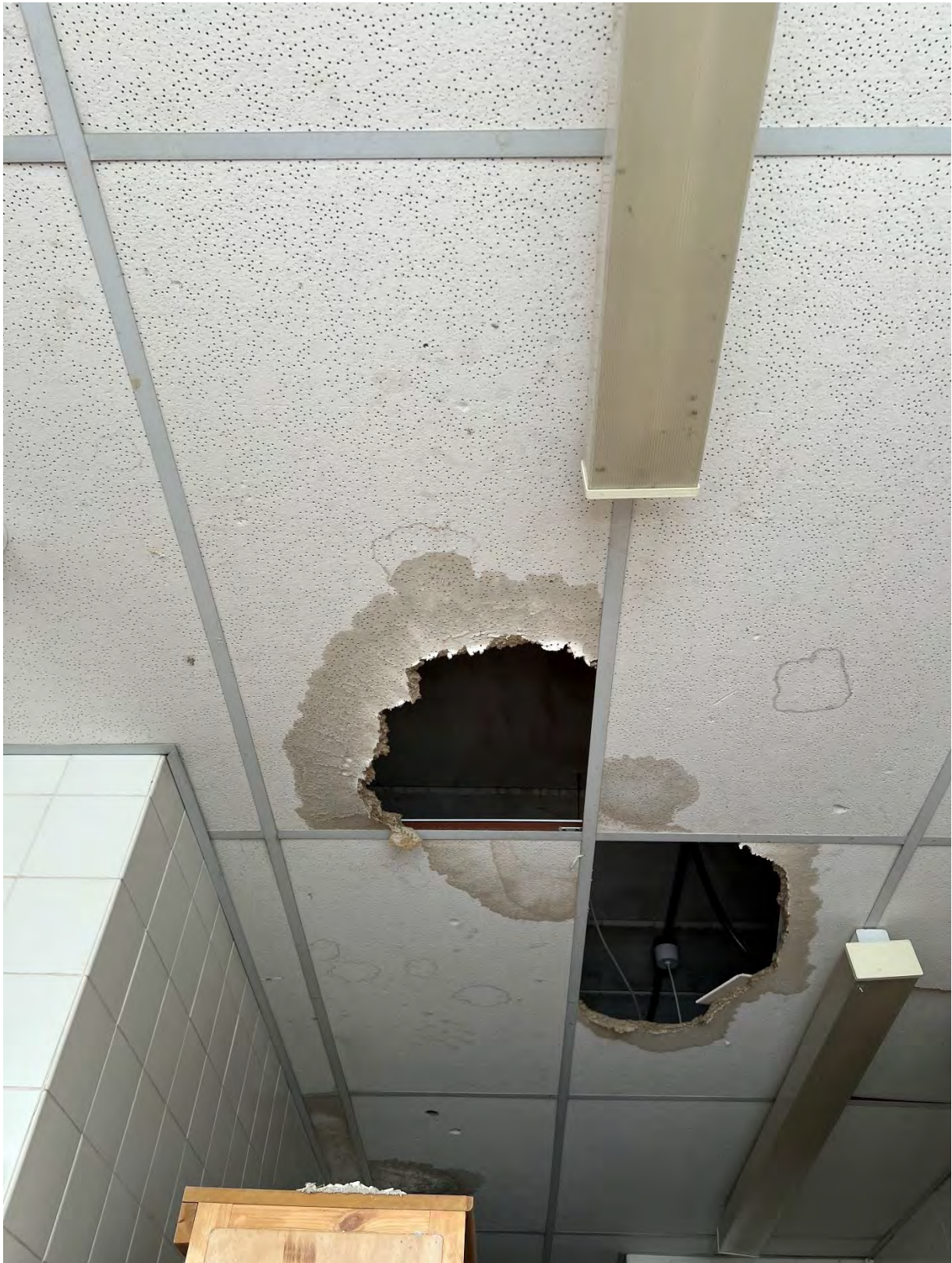
Photo N.13 - Visible water staining on Siporex panels (Science Dept toilets)
