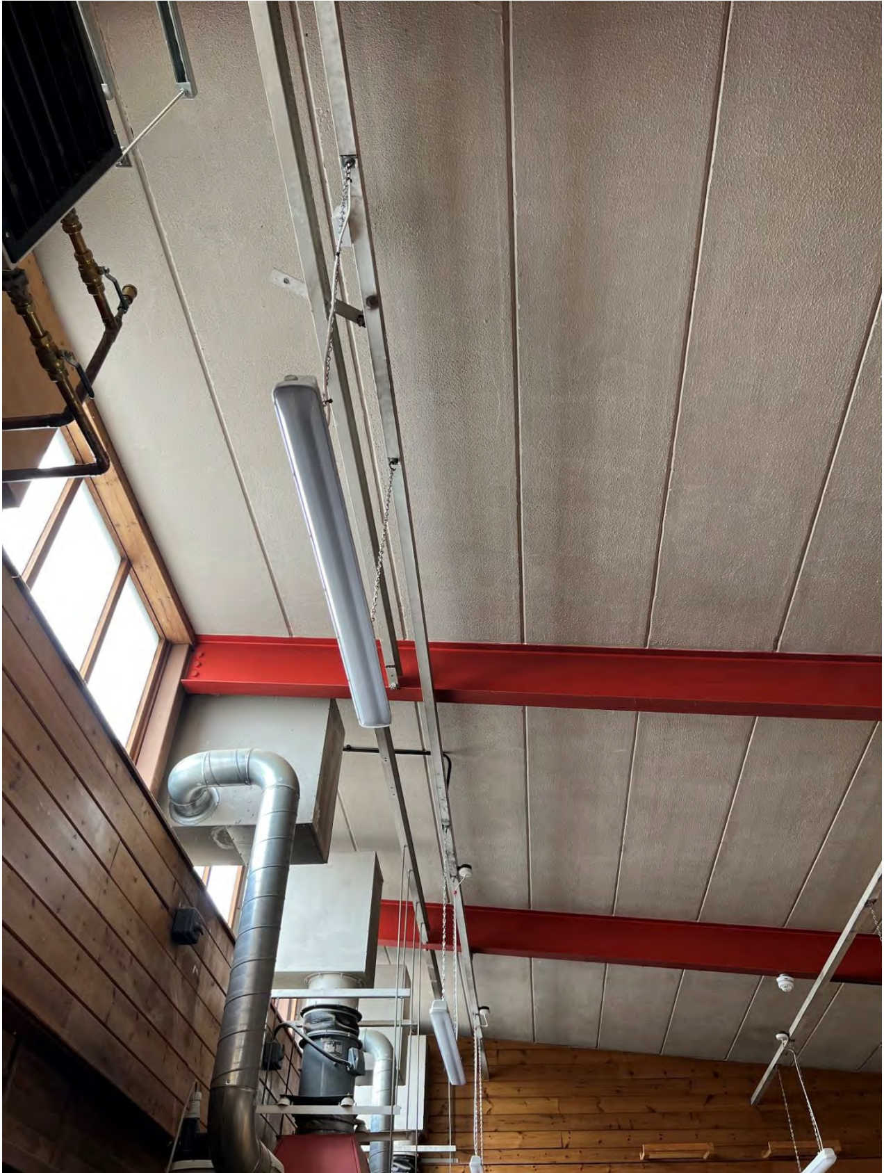
Photo N.2 – Bearing length appears to be less than 75mm throughout (Tech Dept)
