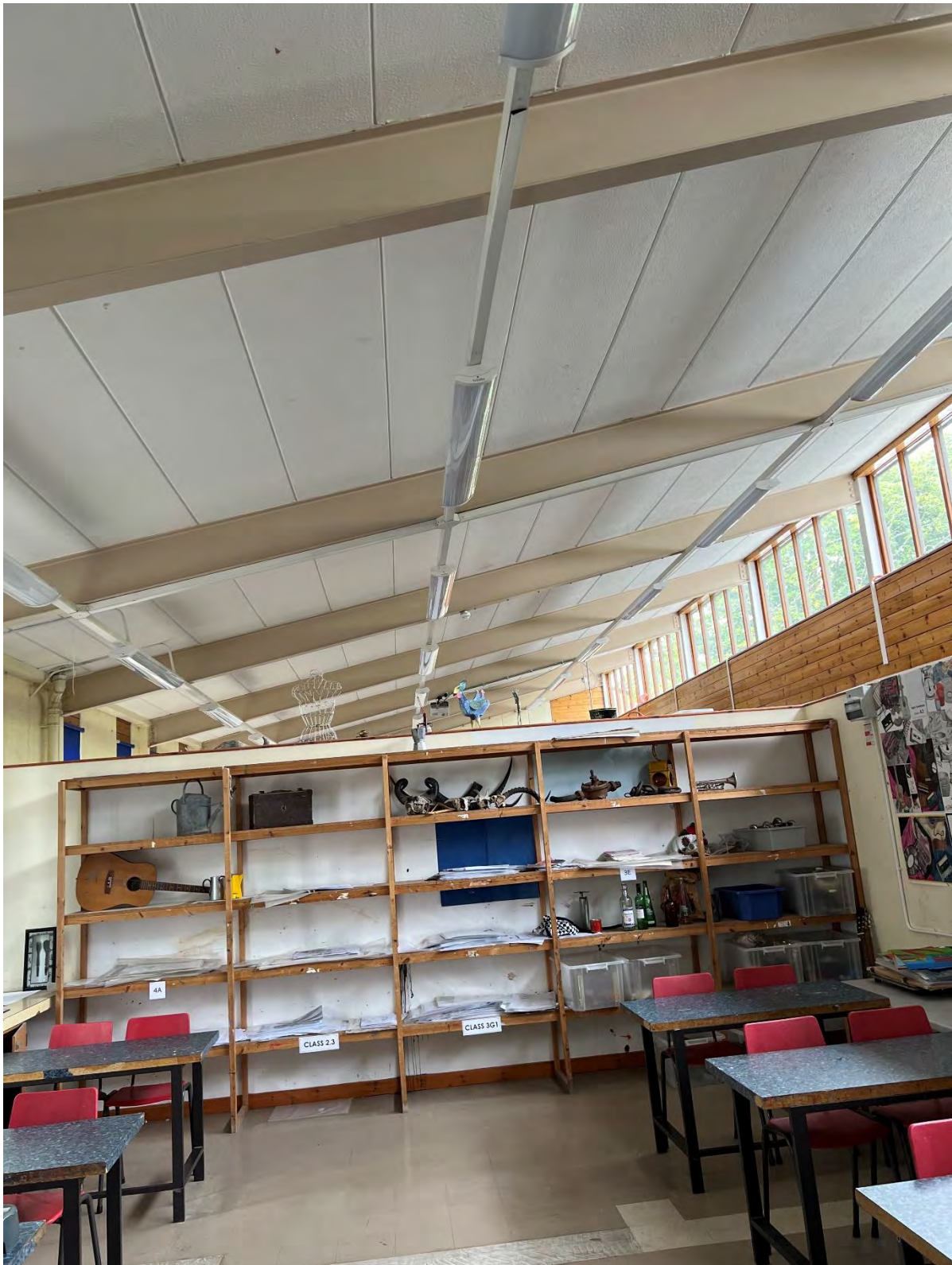
Photo N.6 - Bearing length appears to be less than 75mm throughout (Art Dept)
