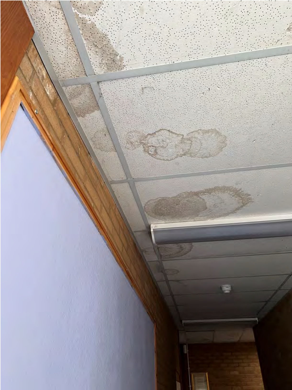
Photo N.11 – Water staining on ceiling tiles indicates potential water ingress (corridor to Home Economic Dept)
