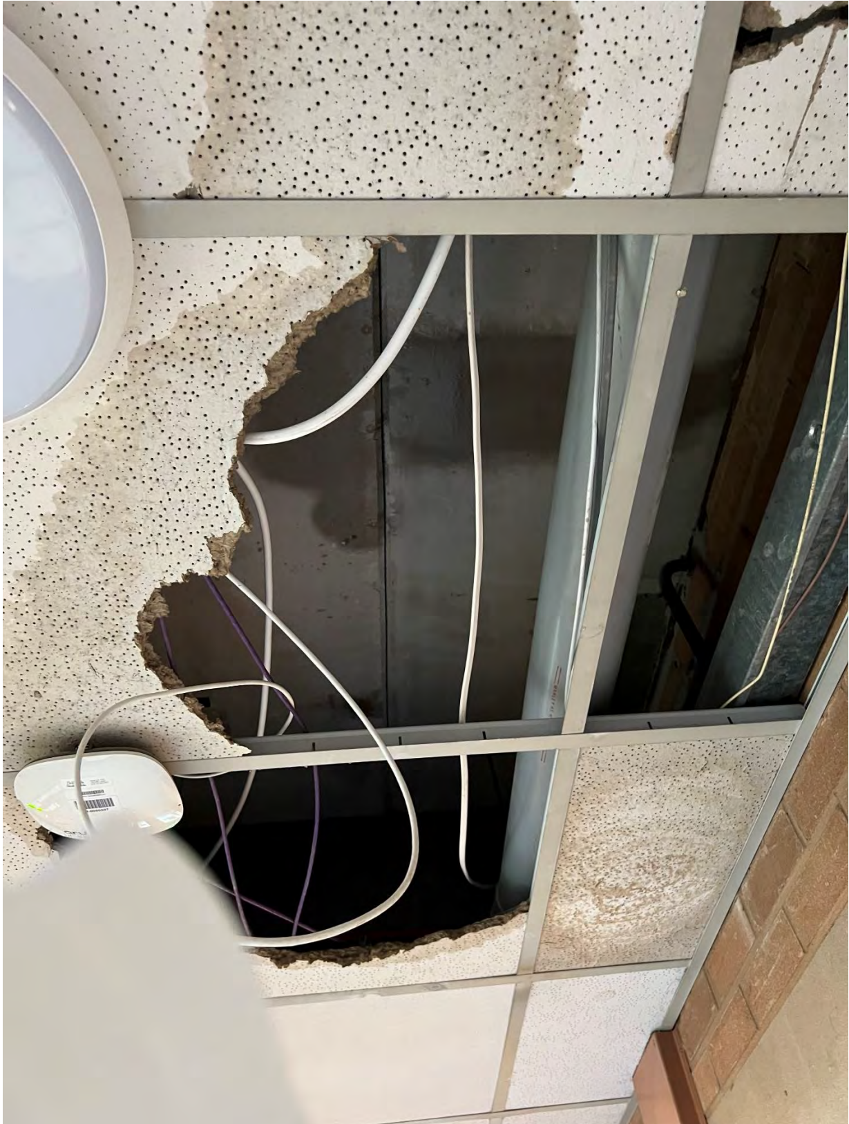
Photo N.12 – Visible water staining on Siporex panels (Science Dept)
