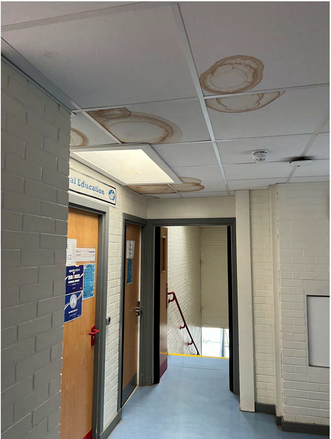
Photo N.16 – Extensive water staining to ceiling tiles (Admin area)
