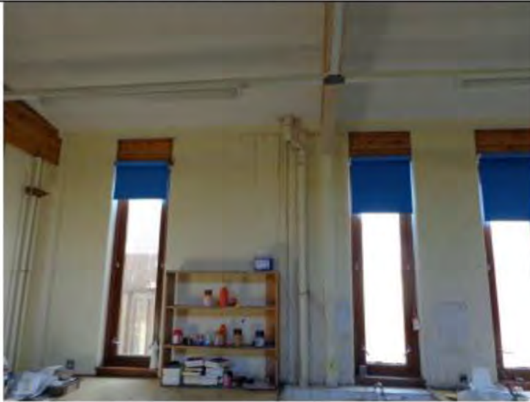
Photo No 4 – Evidence of leaking at rainwater downpipes
