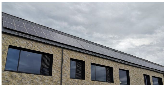
Solar PV panels and natural ventilation. Photos by The Highland Council
