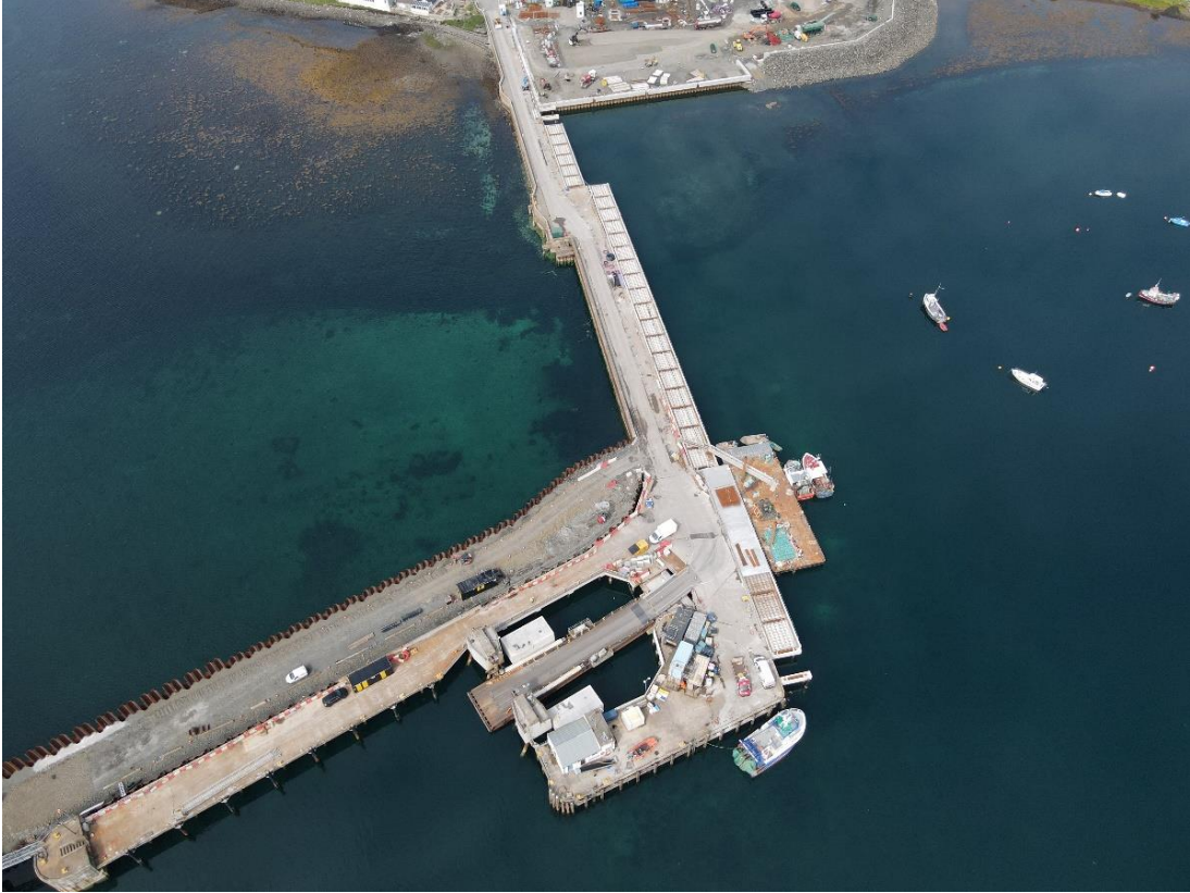
Linkspan Lifting Dolphins and Bankseat
