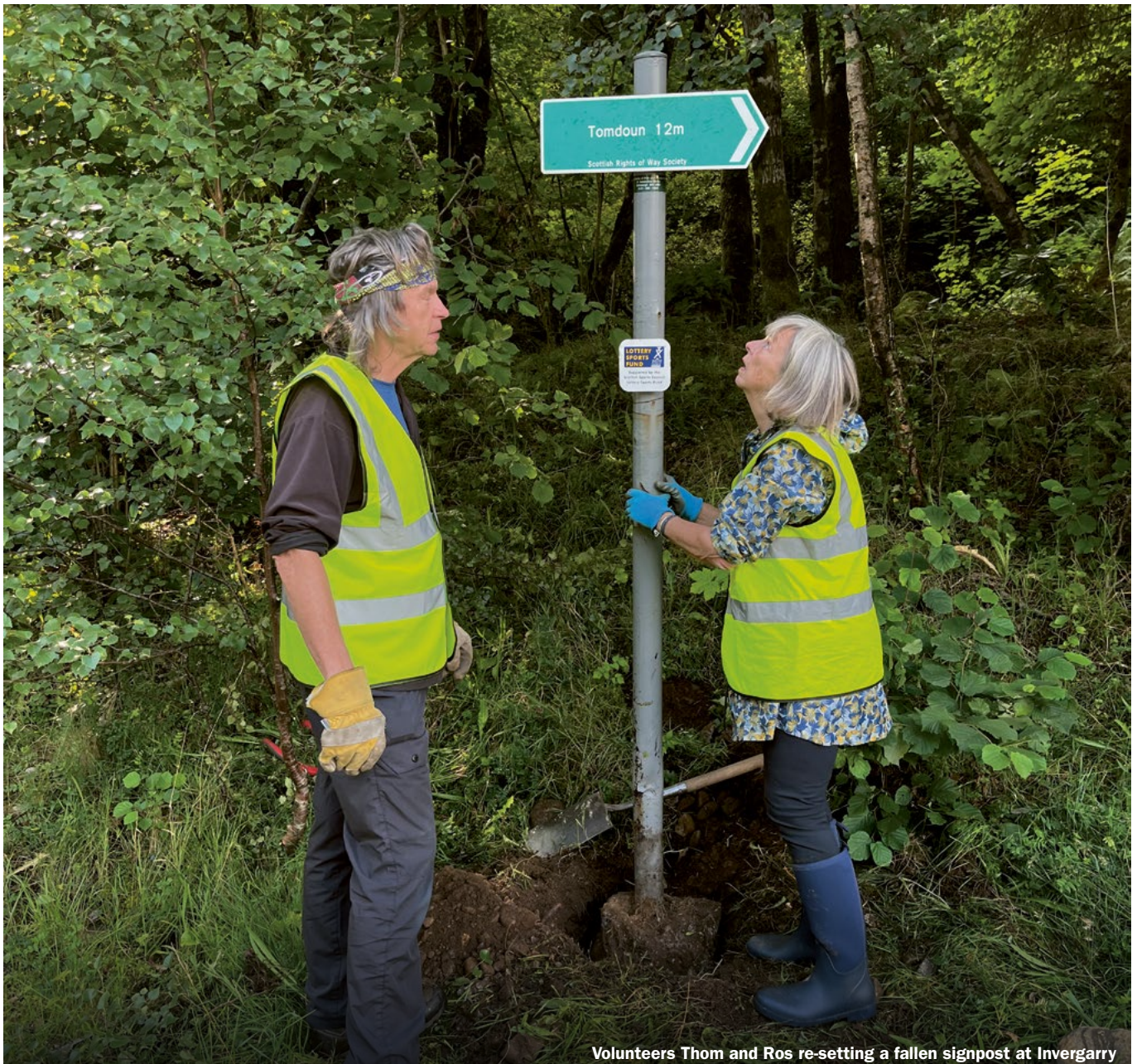
Storm Gerrit damaged our signs in Glen Feshie
