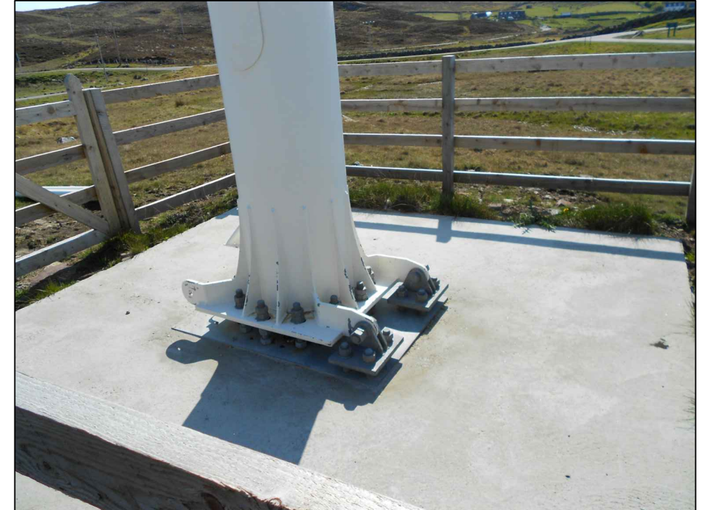
View of Turbine base
