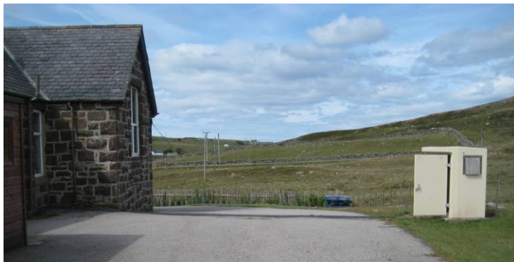
Figure J10-wind turbine external control box at the rear of the school building
