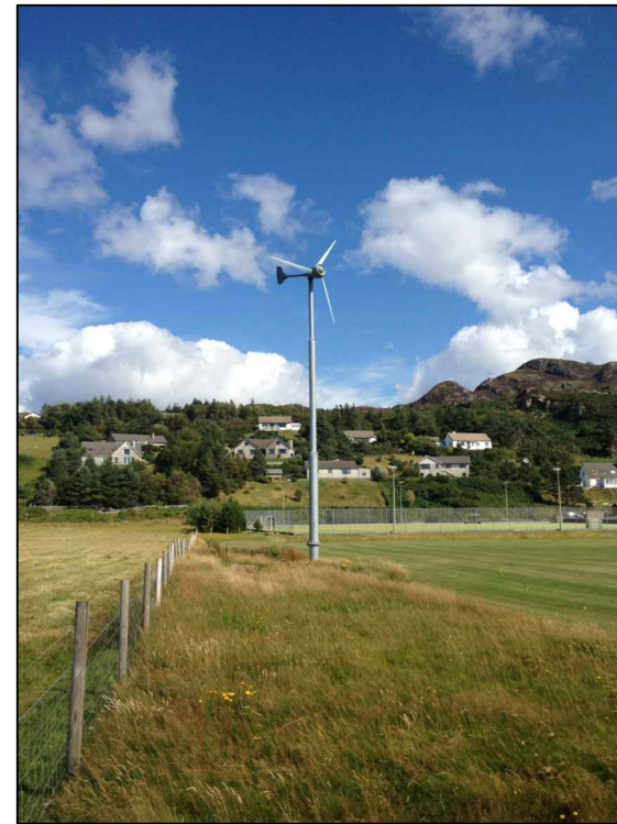
View of Turbine (looking east)
