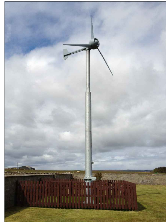
View of Turbine (looking east)
