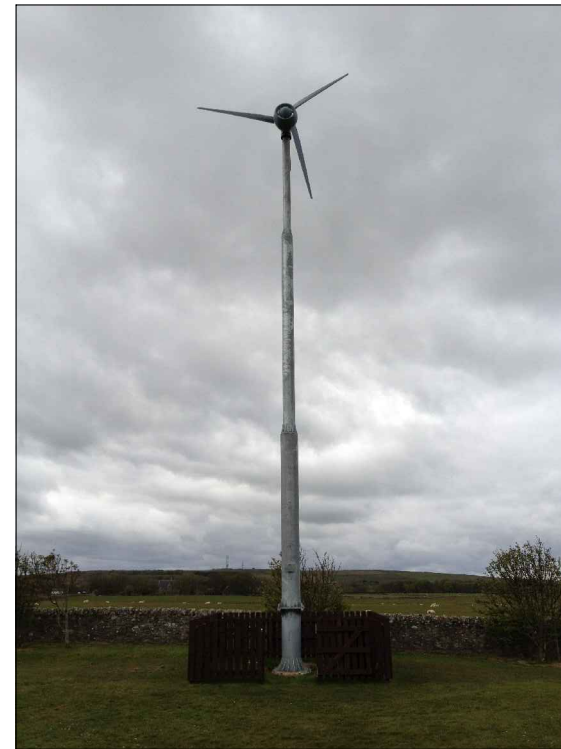
View of Turbine (looking west)
