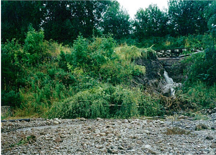
Figure 8-7: Flood from the Railway in September 2002 to Murray Terrace
