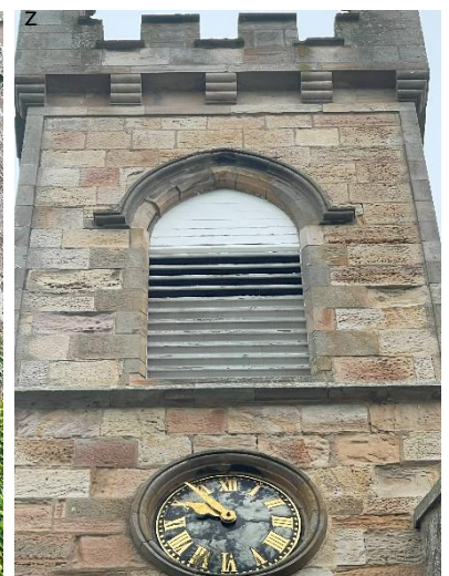
Stonework defects and weathered clockface
