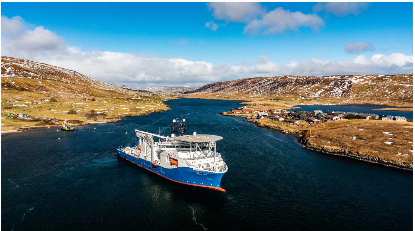
An SSE Transmission vessel prepares to pull an HDVC cable to carry electricity from Shetland to mainland Scotland.
