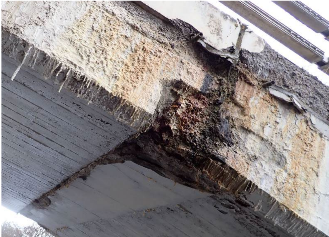
Condition of half joint (February 2025)
